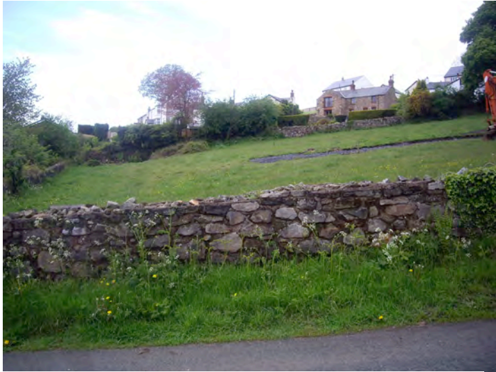
Existing boundary wall to be repaired as required
