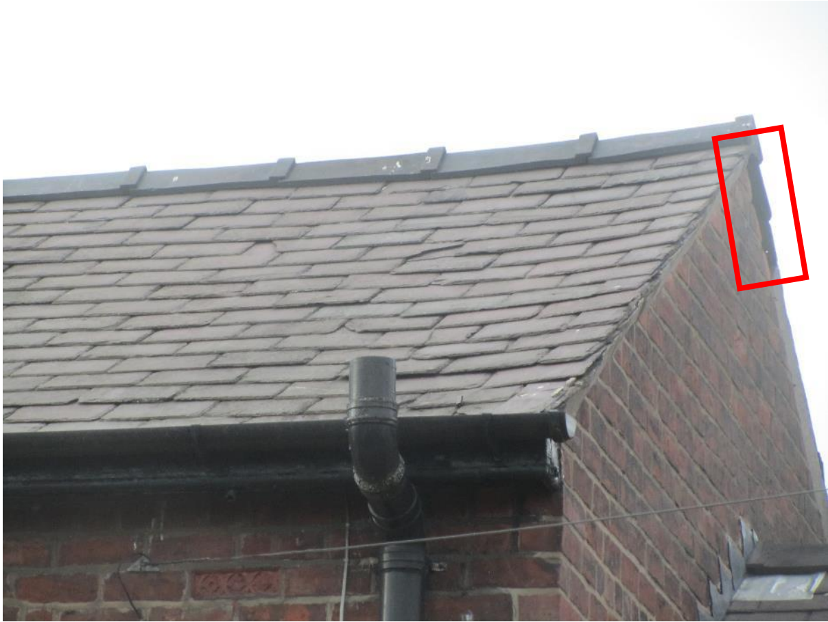
Image 3.18 Mortar gap on an eastern gable wall of B1 (indicated) – considered superficial – also showing slightly broken slates – also considered insignificant
