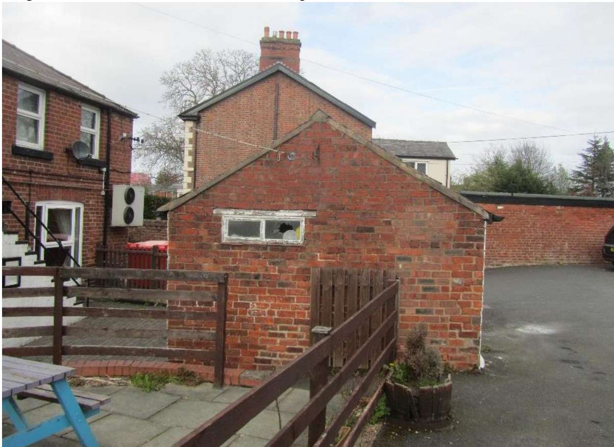
Image 3.22 Western elevation of B2, also showing broken window
