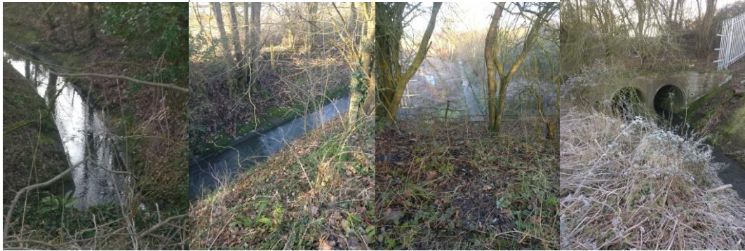
Figure 3 - Redwither Brook - Heavily Modified Channel and Culvert
