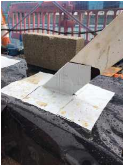
Steel brace fully sealed with
