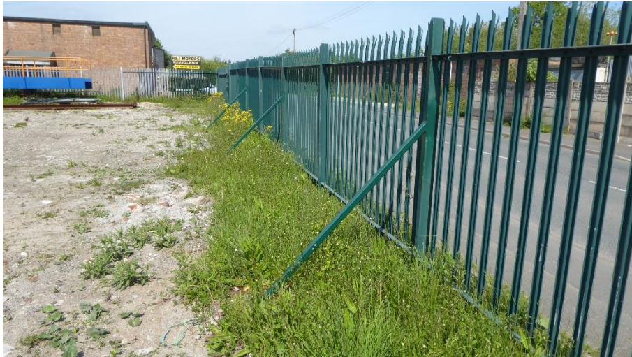
Figure 4.3 Palisade fencing along north western and north eastern boundary
