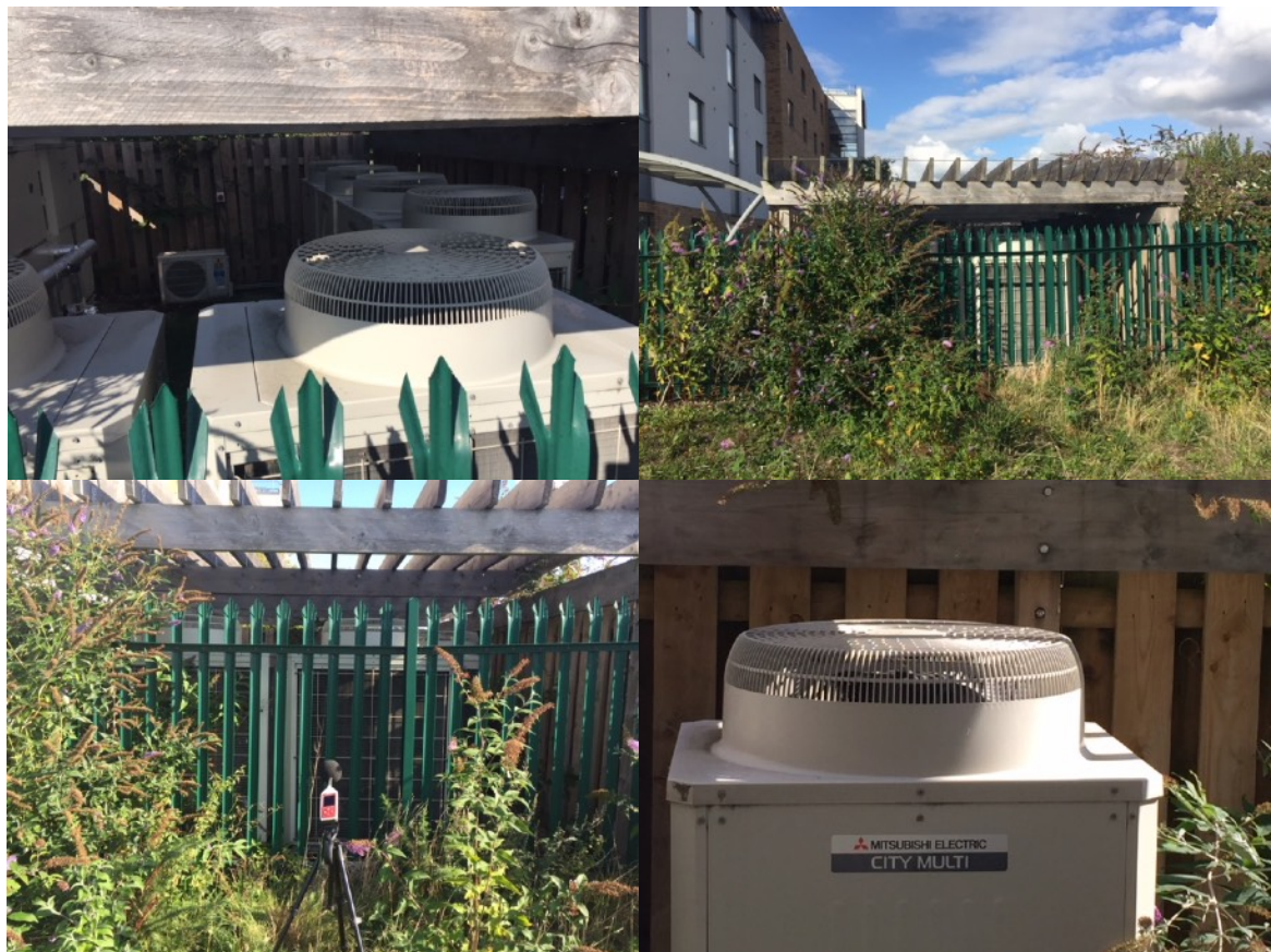
Figures 7 - 10 : Premier Inn plant
