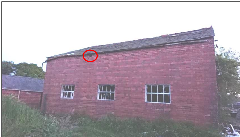
Emergence point at Building 3 - from crevice in brickwork at wall plate
