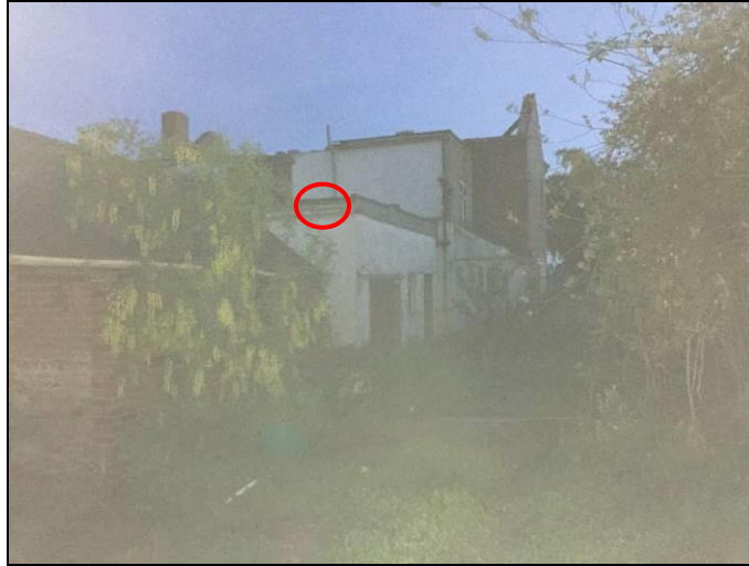
Emergence point at Building 1 - beneath a timber fascia on the single-storey section
