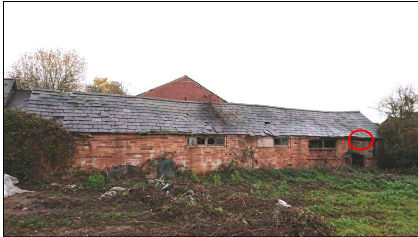
Emergence point at Building 2 - from inside dilapidated barn open door compartment
