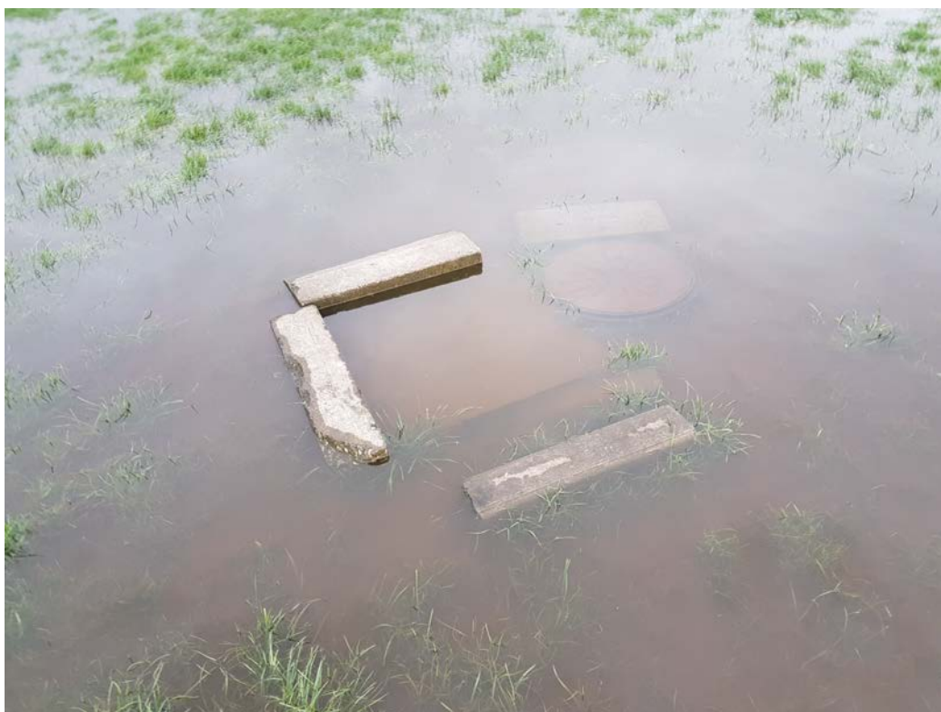
Photo 22 – View of manhole in patch of waterlogged ground in area 4
