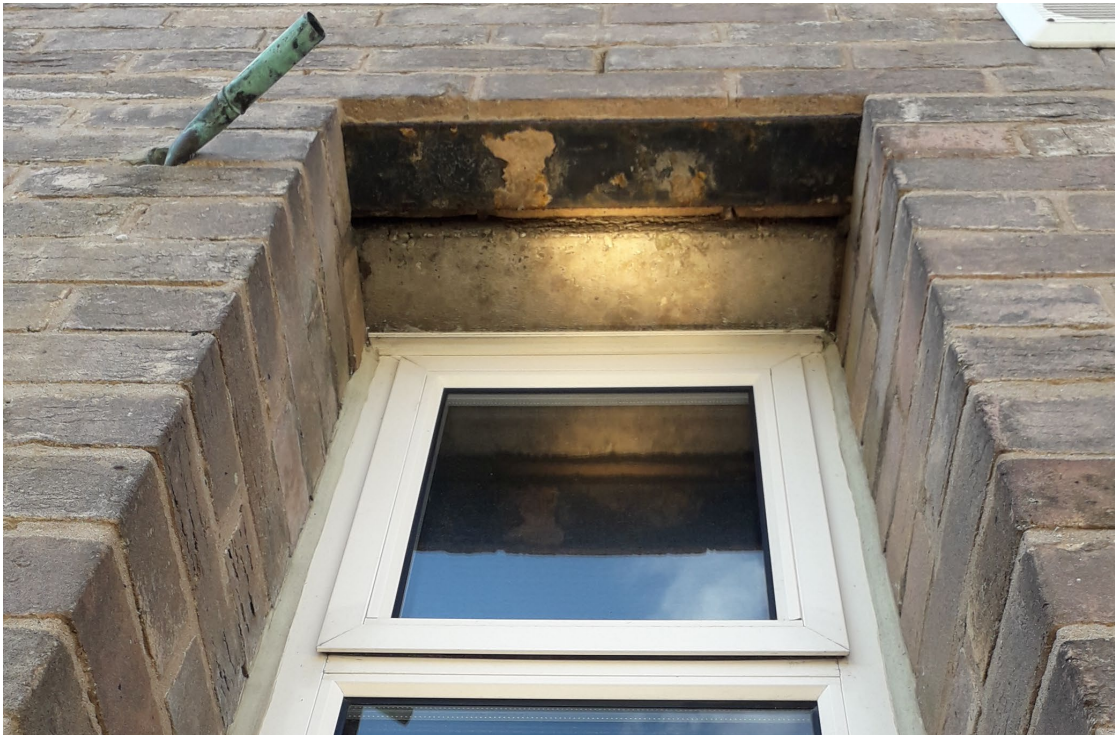
Image EDP 3.5: Gap in concrete lintel at Building 9, north-eastern aspect
