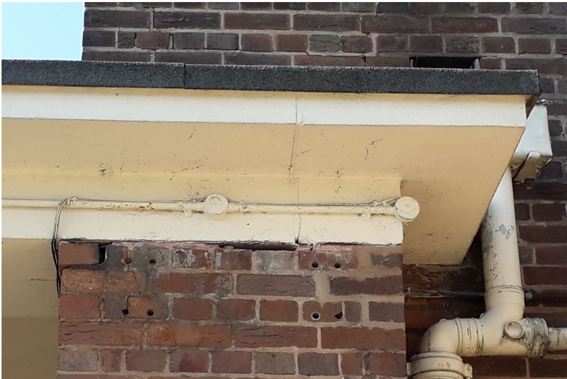
Image EDP 3.4: Hole under soffit on Building 9, north-eastern aspect
