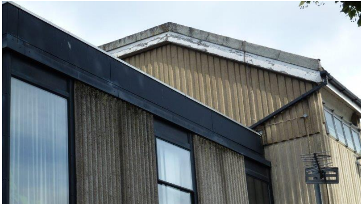
Photograph 6: View of timber barge boards to gable end sports facilities building.
