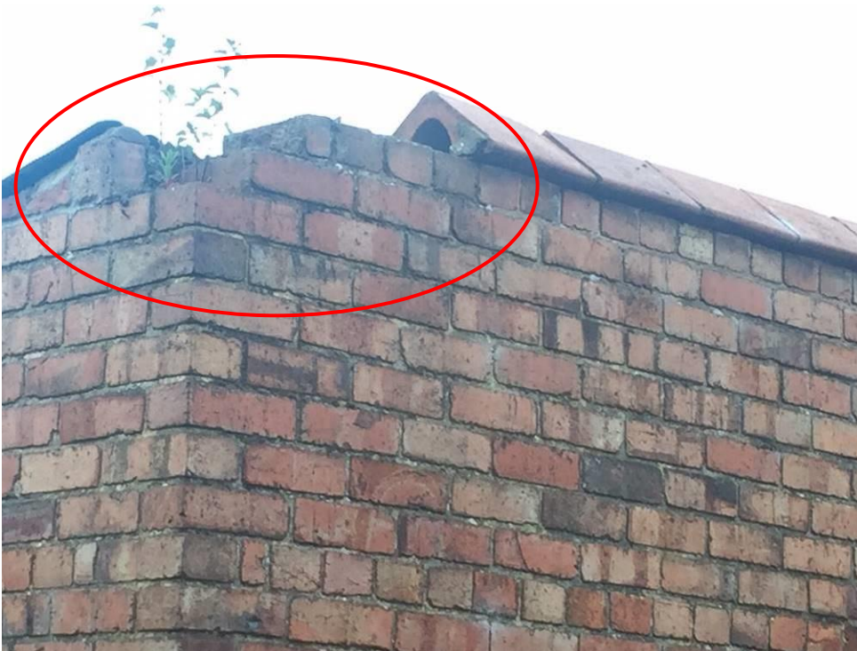
Plate 4: Close-up view of the missing ridge tile.
