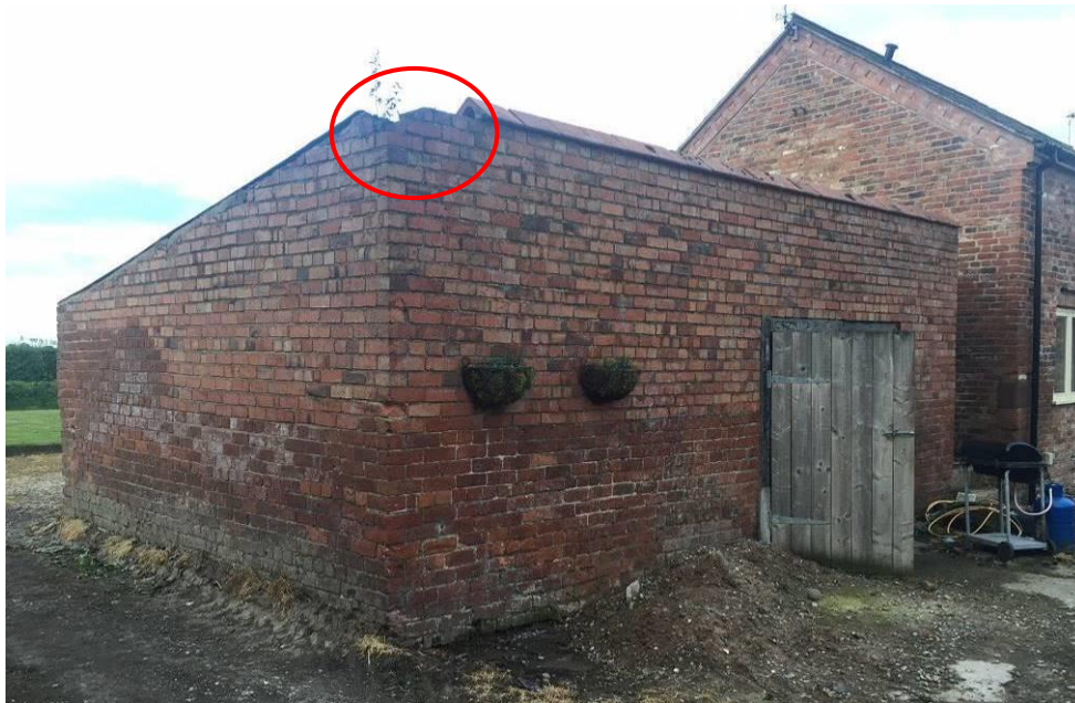
Plate 2: North-east elevation of garage showing missing ridge tile.
