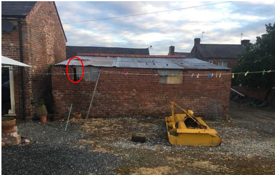
Plate 1: Southern elevation of garage showing gaps in the boarded-up windows.
