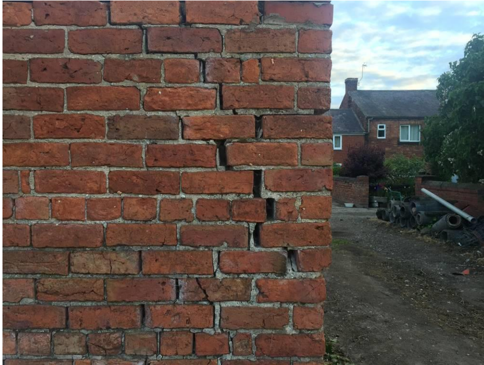
Plate 5: South elevation where the brick-work has slipped out of alignment.
