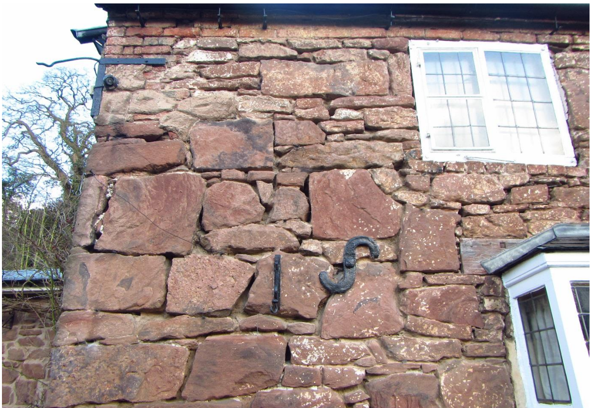
Photo 4. Gaps in the stonework on the southern elevation of Building A.
