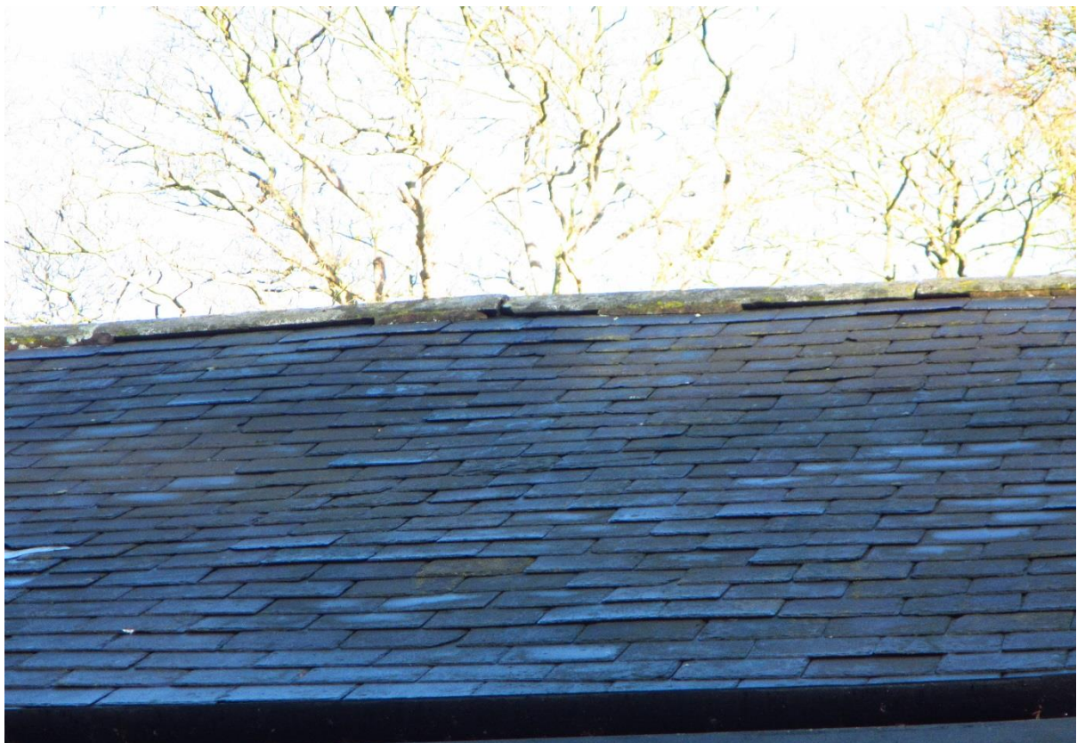
Photo 2. Gaps under ridge tiles of Building A.
