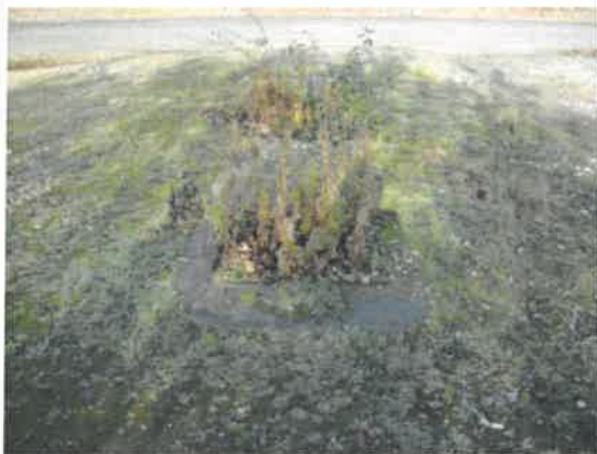
Underground storage tank(s) in entrance way to Unit 226
