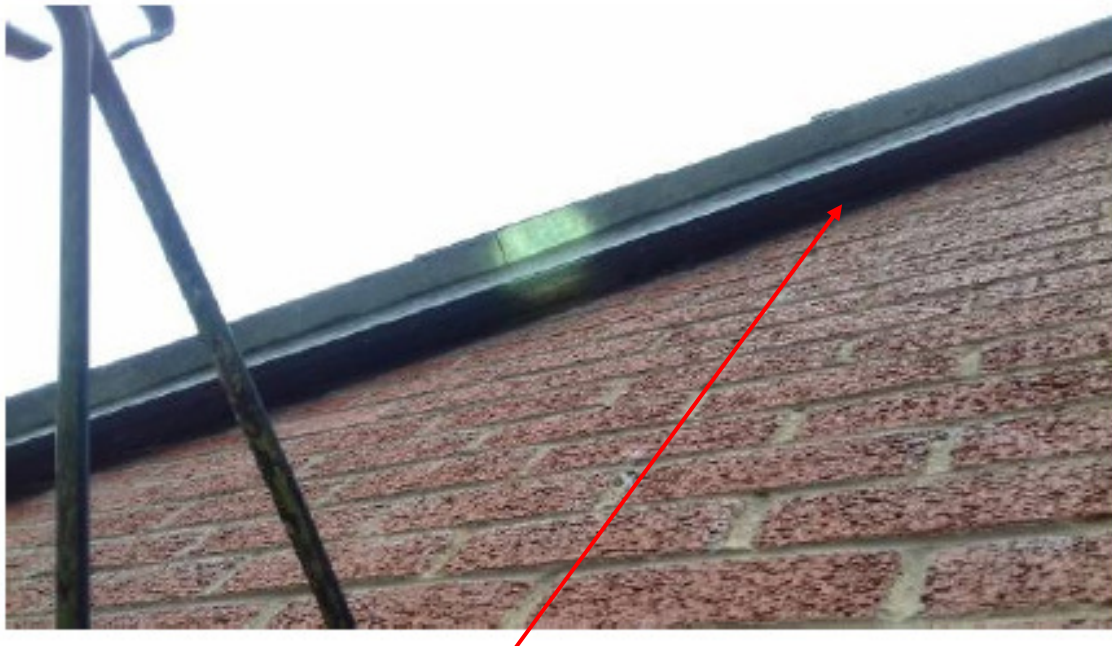
Potential ingress points at western elevation soffit
