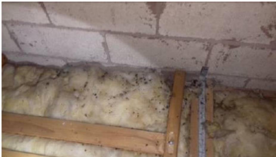
Accumulation of Pipistrelle droppings at internal west gable elevation
