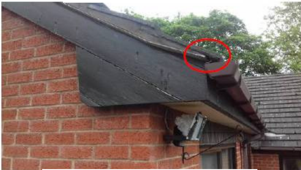
Potential ingress gap at western elevation roof verge
