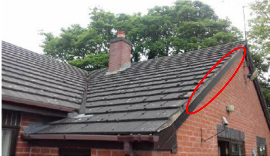
Figure 7: Location of emergence from under soffit board of residential building
