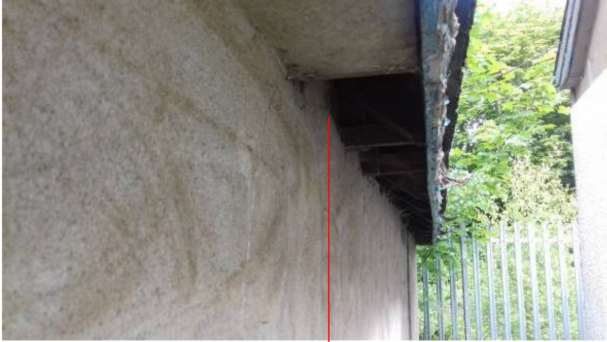
Gaps in soffit of B2
