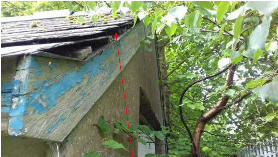
Gaps in the roof verge within B2
