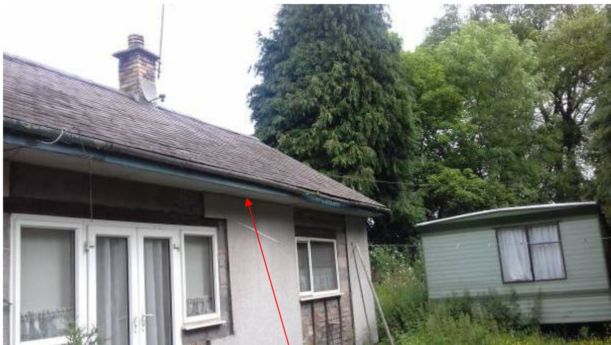
B1 showing gaps at wall plate level and in cement panelling
