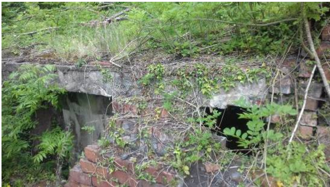
Ingress into areas of B5 via cracks and crevices within brickwork & hibernation potential
