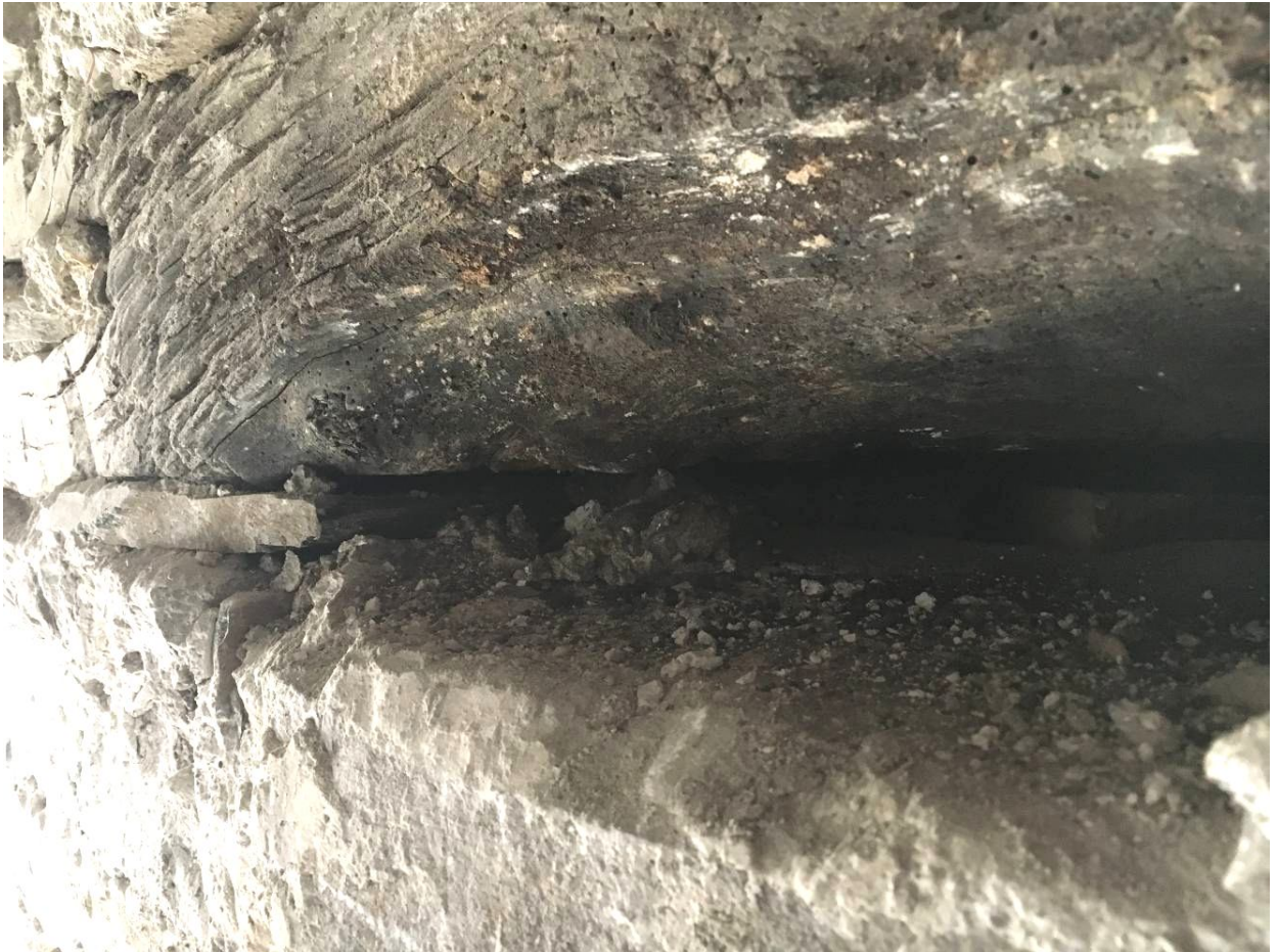
Photo A: Droppings consistent with those produced by brown long-eared bats located below bathroom chimney lintel.
