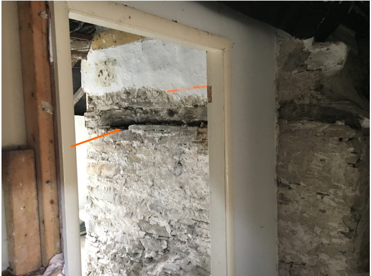
Photo B: Bathroom chimney lintel crevice.
