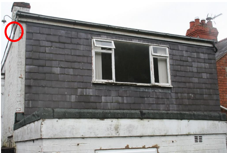
Figure 4.7: Exposed plastic fascia board circled in red
