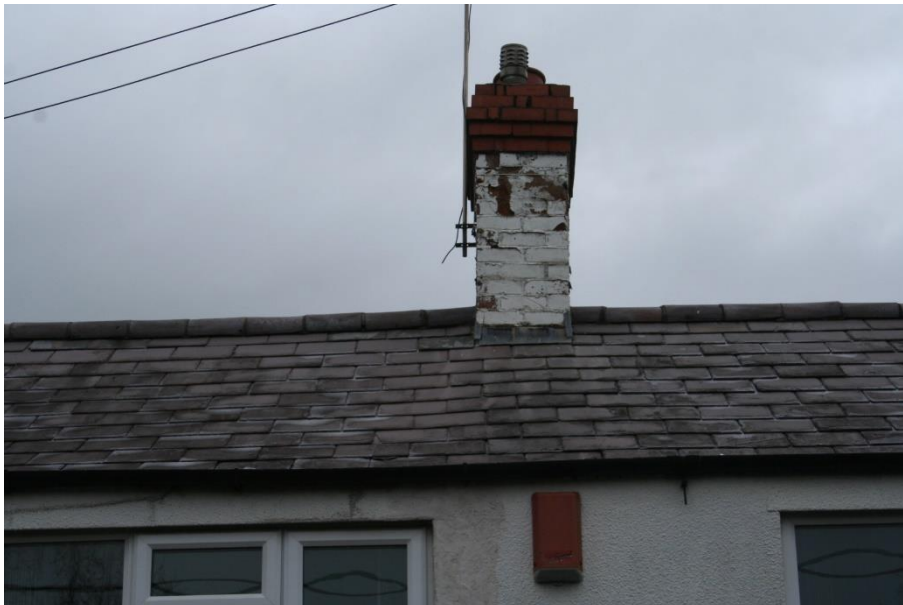
Figure 4.5: Raised ridge tile to the west of the chimney, showing continuous gap.
