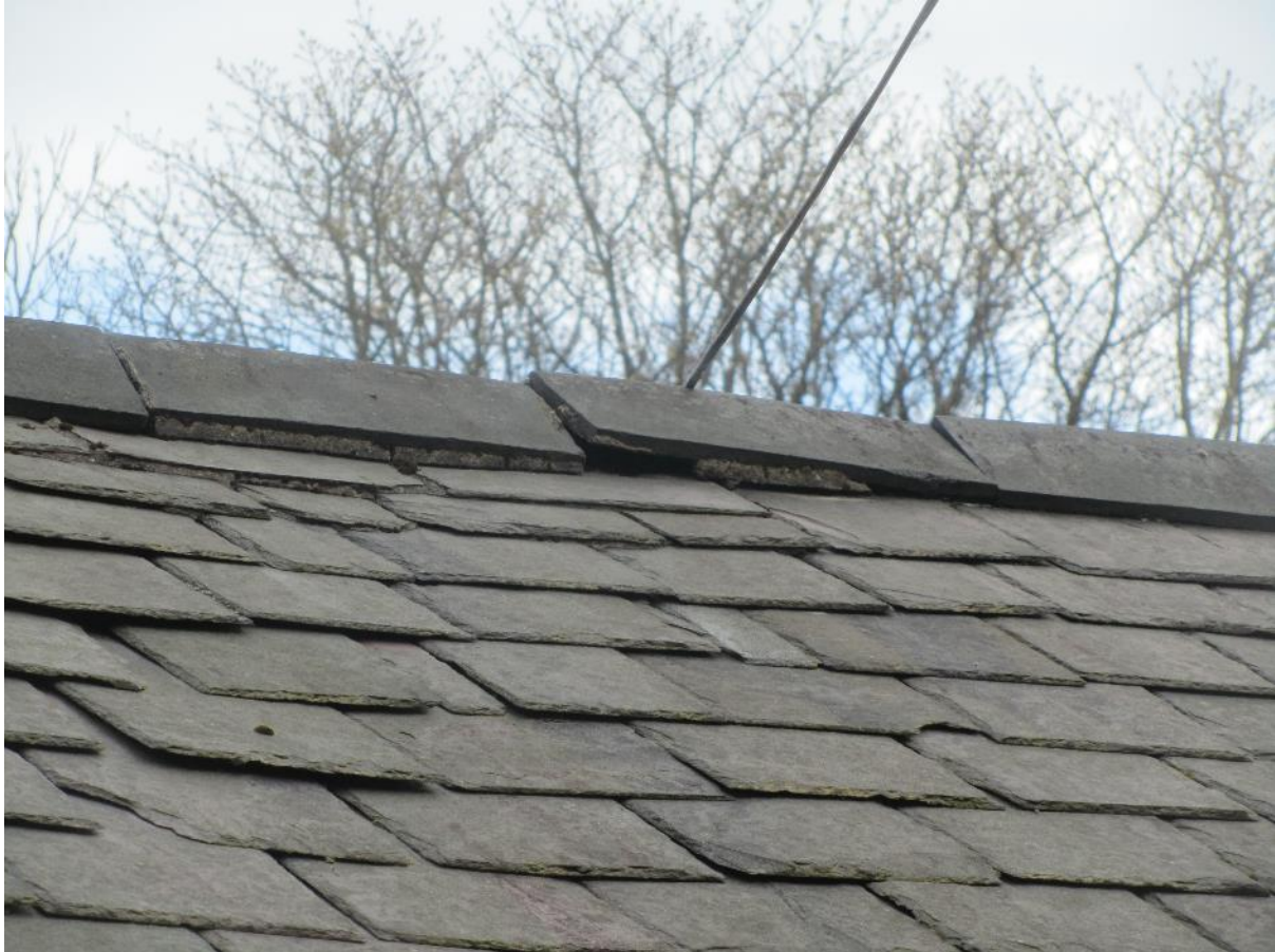
Image 3.23 Ridge tile gap on the northern elevation of B2
