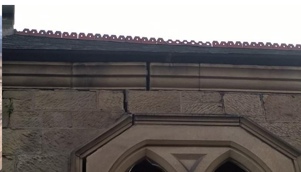
Figures 6 – large gaps between stonework
