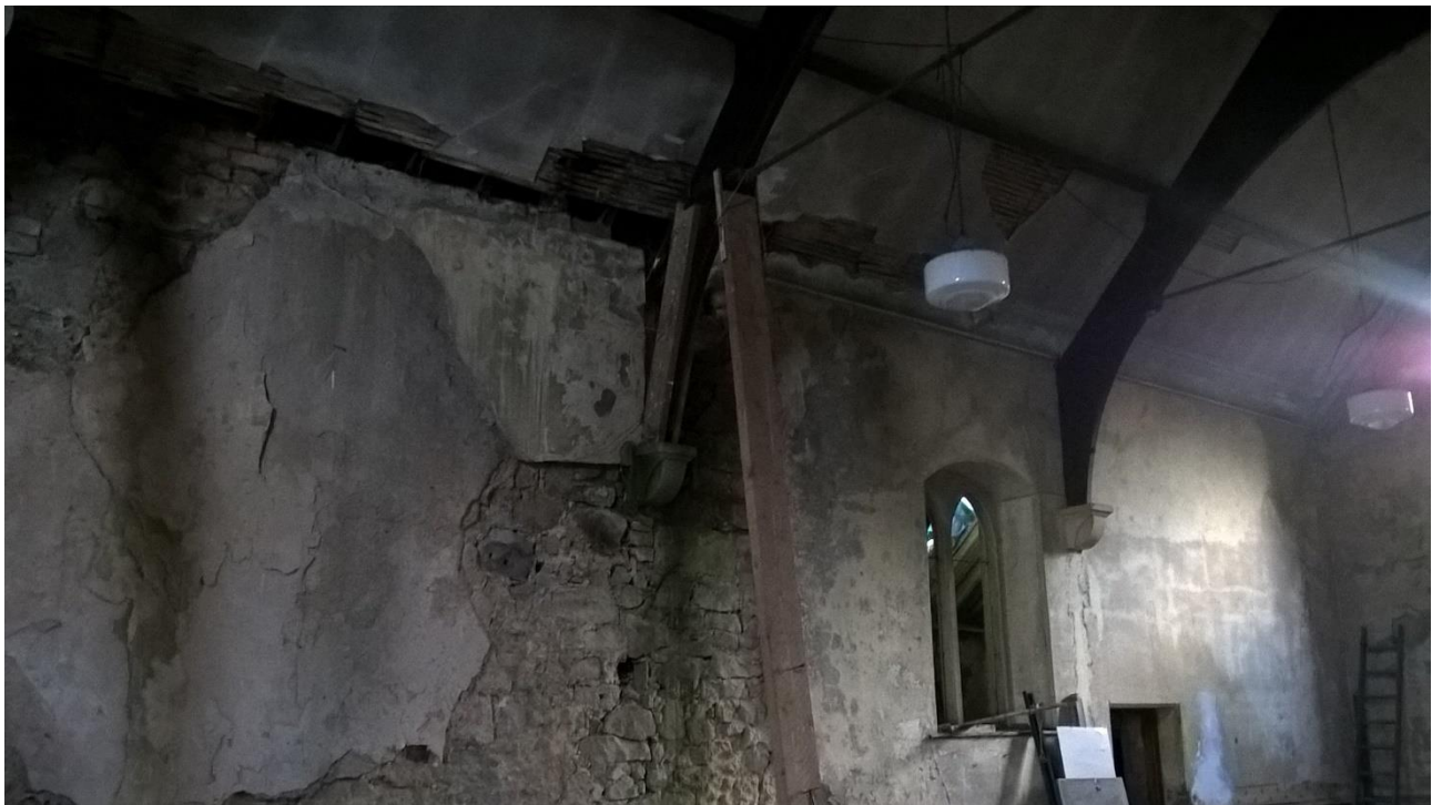
Figure 10 – illustrating the condition of the plaster on the western wall, also the window to the right which leads into the lean-to
