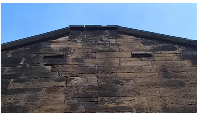
Figure 8 – gaps in stone work
