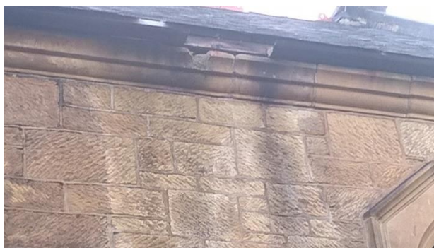
Figures 5 – loose stone where barge board is missing
