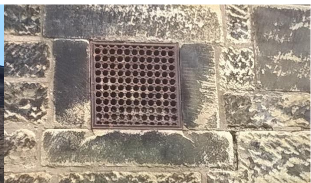
Figure 9 – vents present on the northern side of the building
