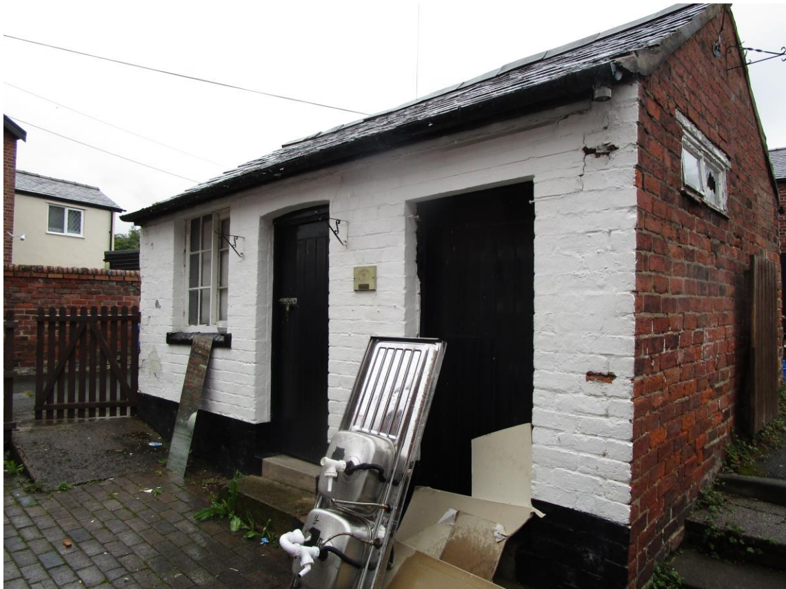
Photograph 13 – showing elevation to out building nearest to public house with cracking evident to top right of right-hand door
