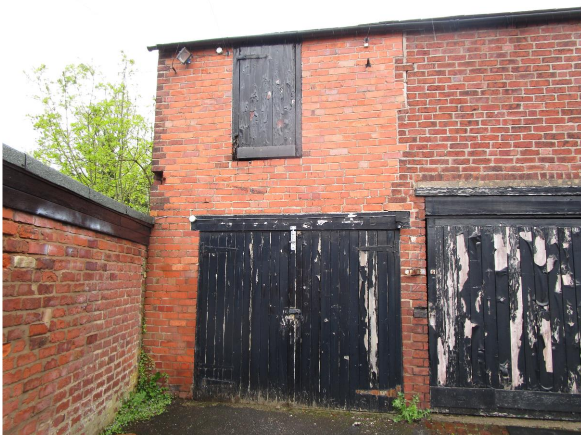
Photograph 2 – showing poorly rebuilt left-hand section of front elevation
