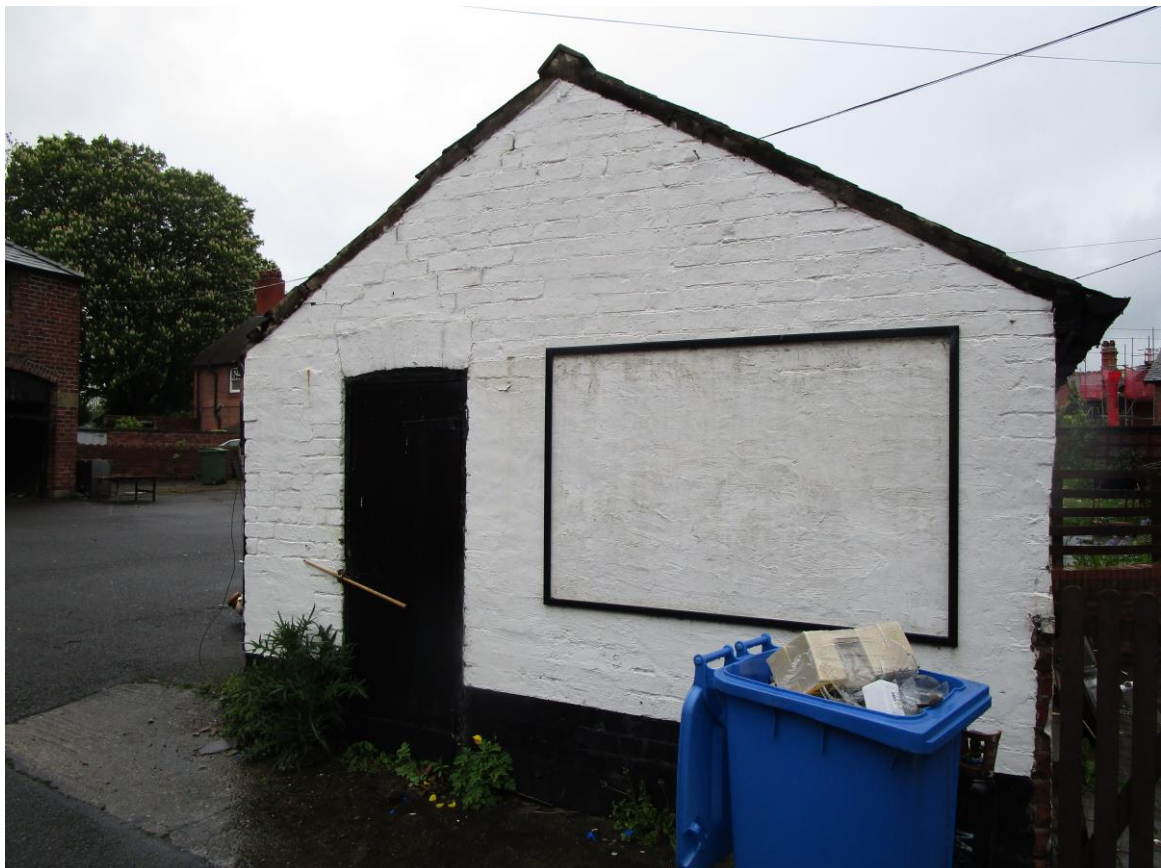
Photograph 12 – detached out building showing minor cracking above the arch to side door
