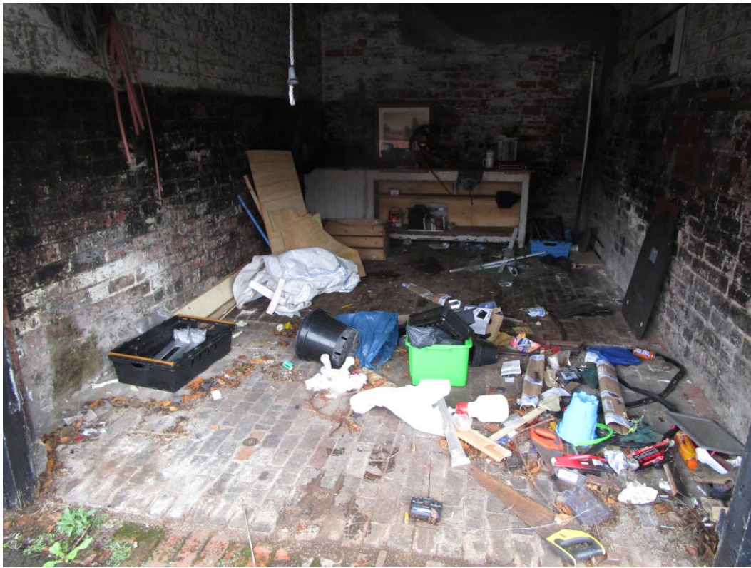
Photograph 9 – showing right-hand stable with paved flooring lacking damp resistance
