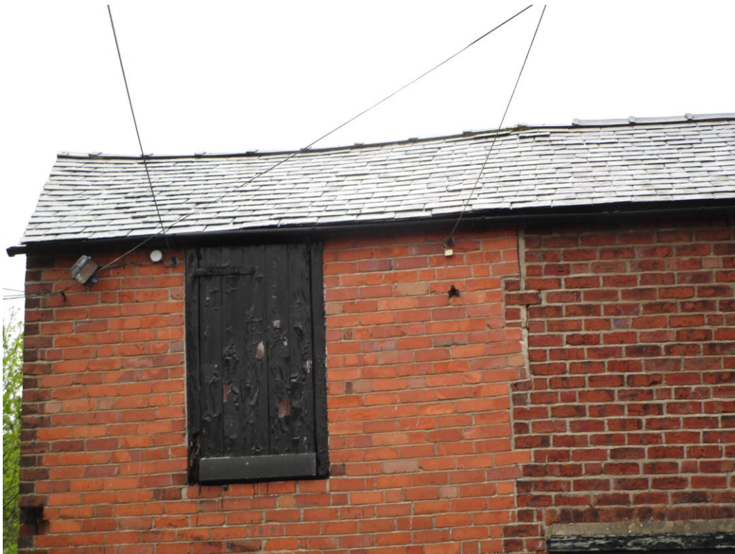
Photograph 4 – showing deflection to roof and separation within brickwork
