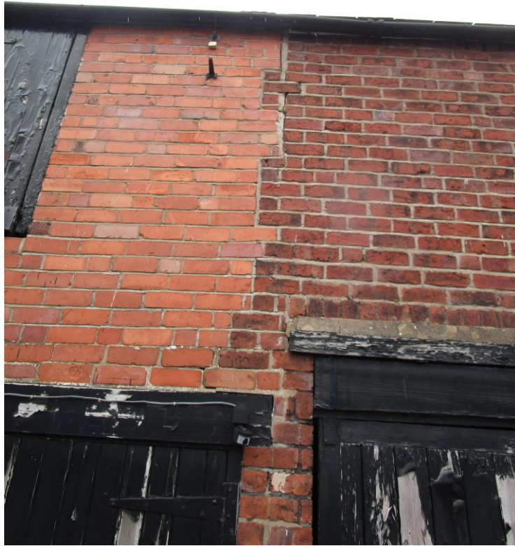
Photograph 3 – showing separation at junction of rebuilt brickwork
