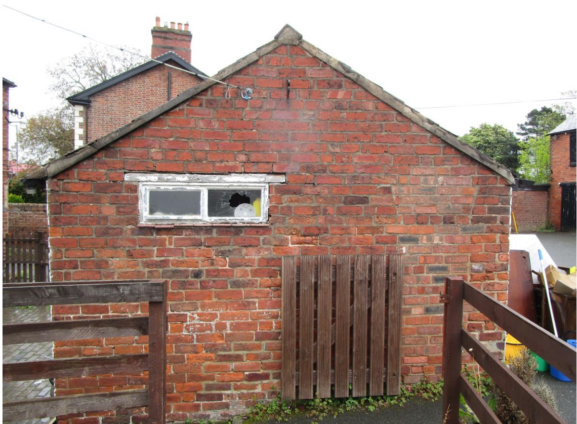
Photograph 14 – showing side wall of out building with brickwork above window inadequately supported and generally in poor condition
