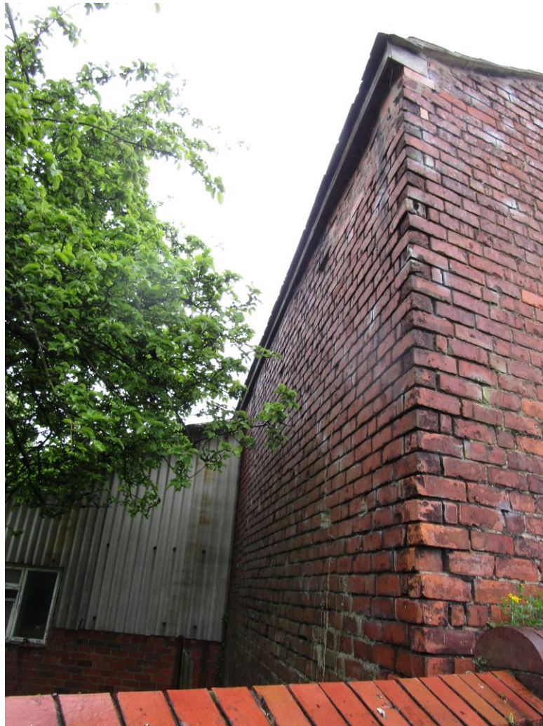
Photograph 7 – showing weathered brickwork to rear left-hand corner and attached outbuilding to rear elevation
