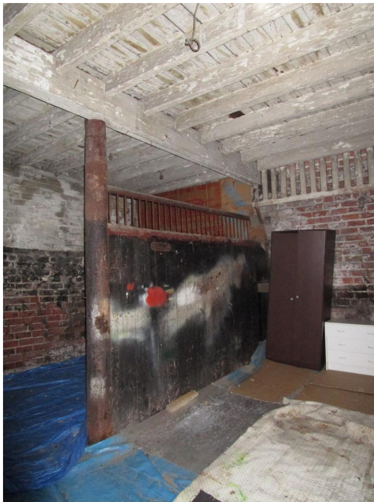
Photograph 10 – showing poor structural arrangement to first floor construction
