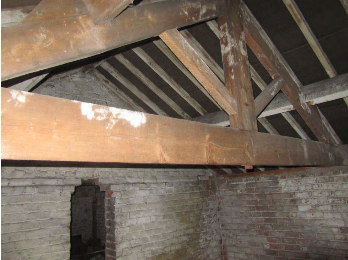
Image 3.28 A typical view within the first-floor level of B3 – showing partition wall with open gap
