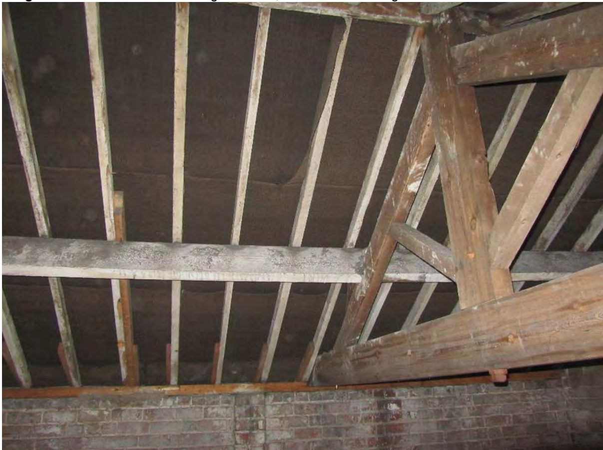
Image 3.29 Bitumastic felt roof lining within B3, with occasional sags noted
