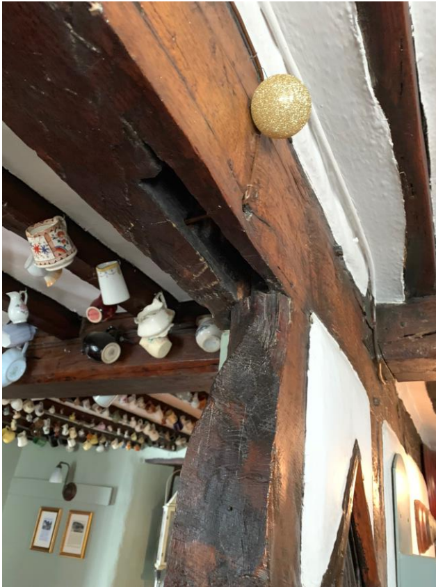
Figure 6- slots visible on lower side of beam, suggesting adapted re-use
