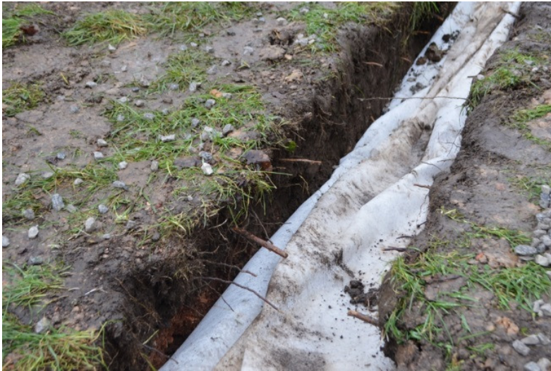
Photo 2. Small exposed roots to T114
