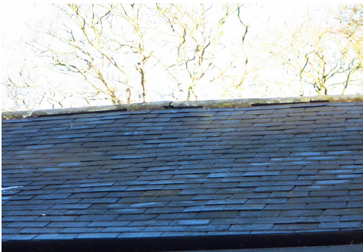
Photo 2. Gaps under ridge tiles of Building A.
