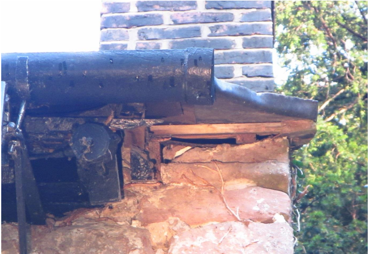
Photo 3. Gap at the eastern corner eaves - Building A.
