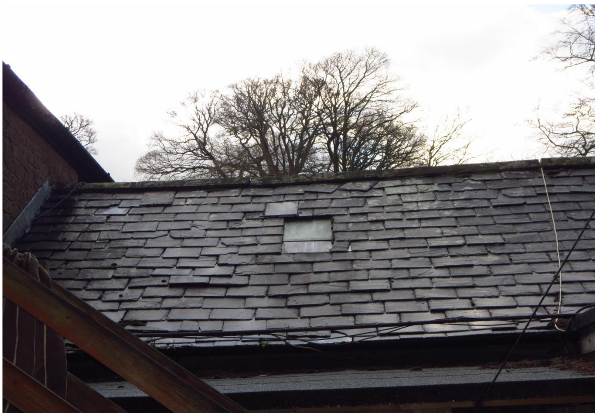
Photo 9. Raised and slipped roof tiles - Building C.
