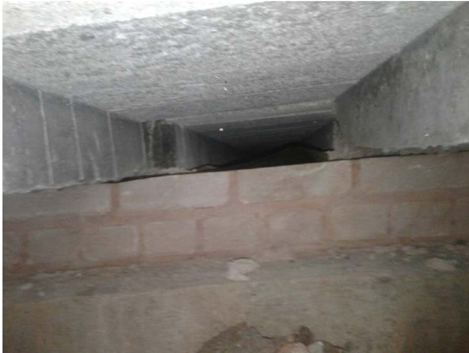
Photograph 2: Approximate 200mm gap through sleeper wall to allow subfloor ventilation (25.07.18).
