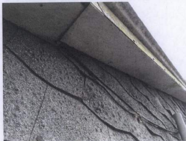
Minor & limited gaps between the soffit and felt tiles
