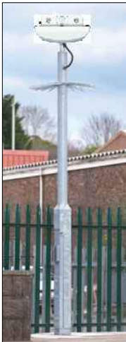
Fig 2. - COLUMN MOUNTED ACCESS POINT (NYS)
