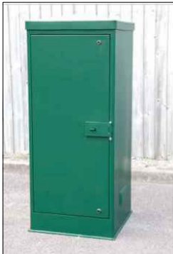
Fig 1. - EXTERNAL COBAGS CABINET (NYS)
