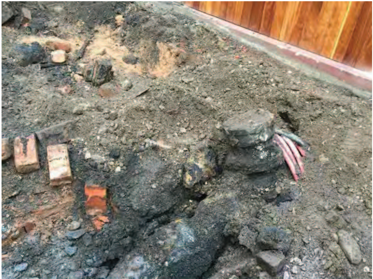
Photo (61): 4No High Voltage electric cables wrapped round redundant gas pipe within Excavation Area 14
