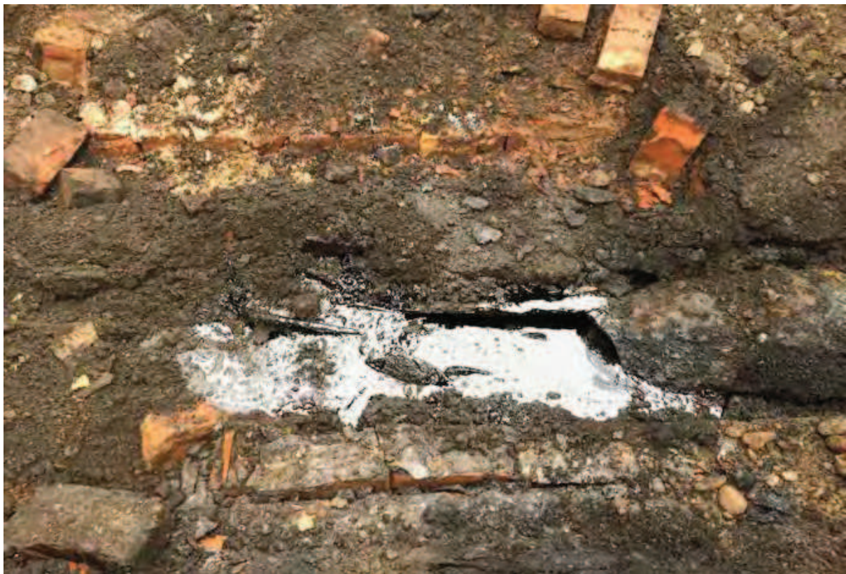
Photo (60): Redundant gas pipe full of tar encountered with Excavation Area 14
