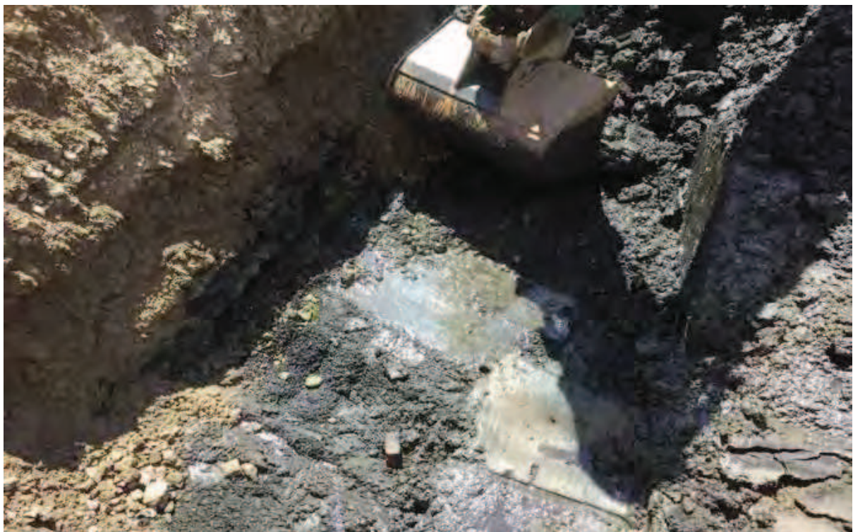
Photo (48): Base of Excavation Area 12 at 2.5m – minimal clay present straight on to sands and gravels with visual evidence of contamination
