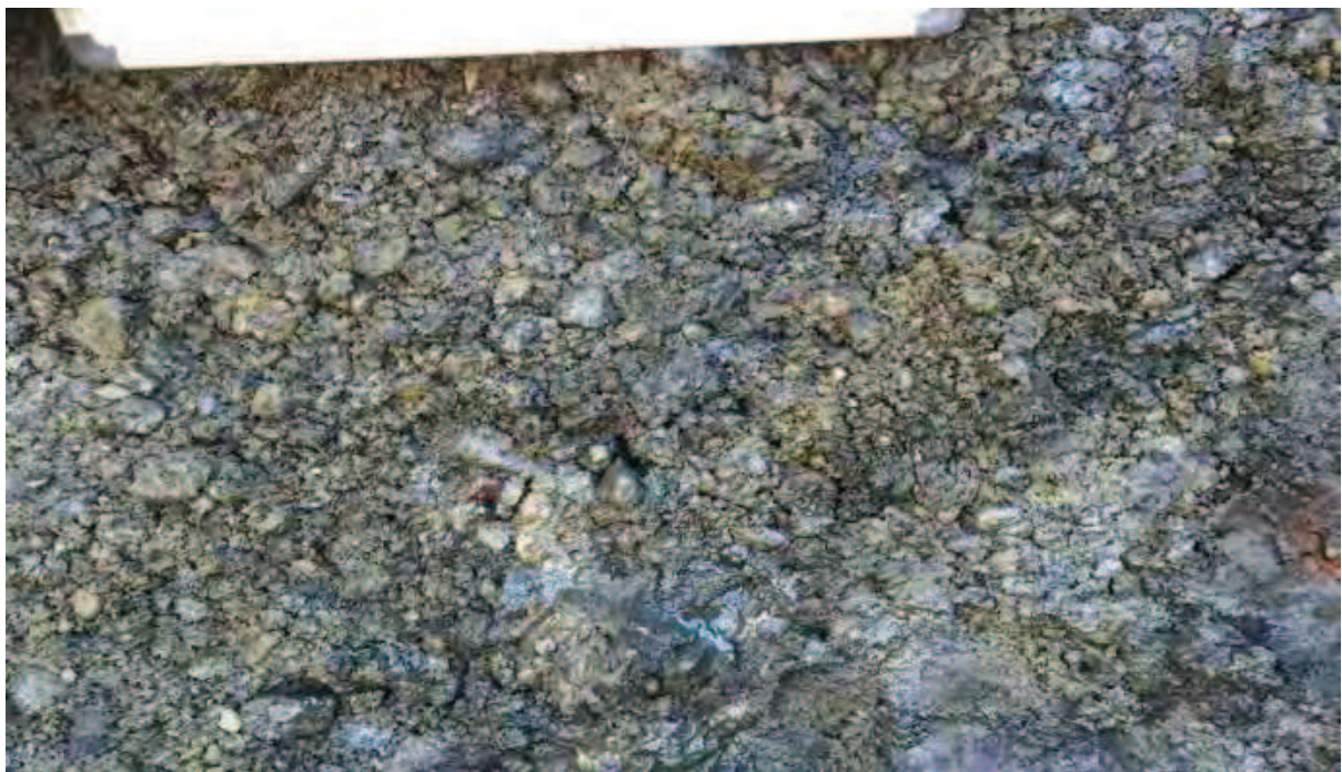
Photo (36): Base of Excavation Area 11 – no clay encountered straight on to sands and gravels, visual evidence of contamination to sands and gravels
