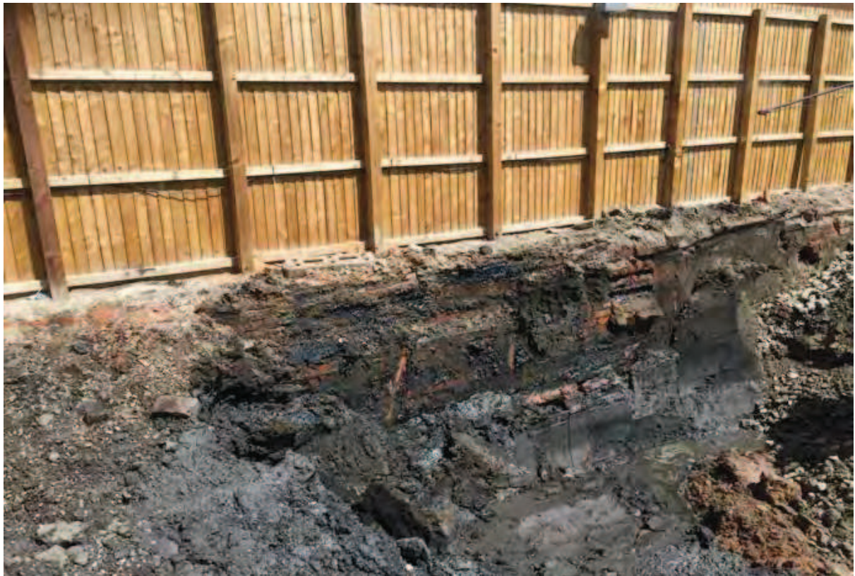
Photo (51): Excavation Area 12 – tar staining to brick work extending under Rivulet Road
