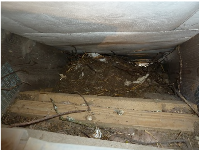
P5: Jackdaw nest in roof space of Building 1.
