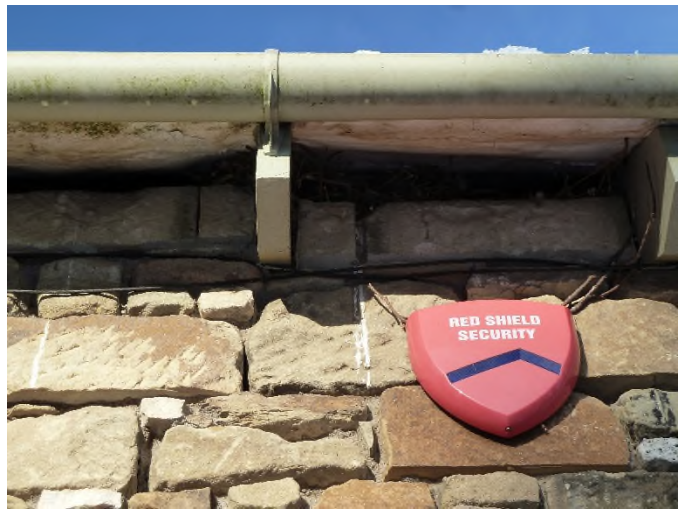
P4: Open eaves and evidence of Jackdaw nesting at southeast elevation of Building 1
