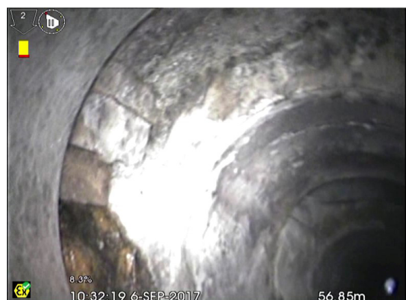
C2X_957cfd90-7a00-4091-8a0f-8d68fef4e719_20170912_082246_721.jpg, 00:06:03, 56.85m Open joint, large
