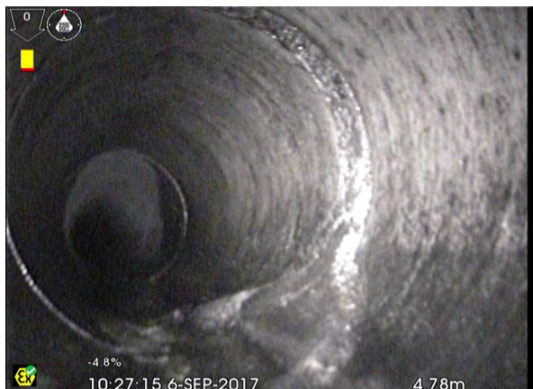
C2X_d2a7c5d0-a28b-47b8-ab8c-a537c3cedf05_20170912_081251_626.jpg, 00:00:59, 4.78m Attached deposits, encrustation from 4 o'clock to 7 o'clock, 3% cross-sectional area loss
