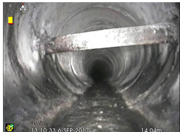
C1X_06a23d8d-747e-412d-b068-9f247a6ee966_20170912_084547_481.jpg, 00:01:38, 14.04m Other obstacles, other from 3 o'clock to 9 o'clock, 10% cross-sectional area loss
