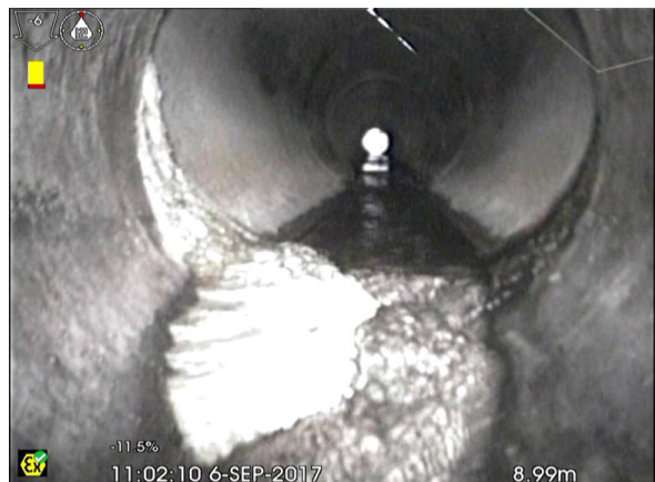
C3_H.wallX_cae23a6f-c0cc-48f1-a634-35f3af4b8d59_20170912_083506_942.jpg, 00:01:40, 8.99m Attached deposits, encrustation from 5 o'clock to 7 o'clock, 5% cross-sectional area loss
