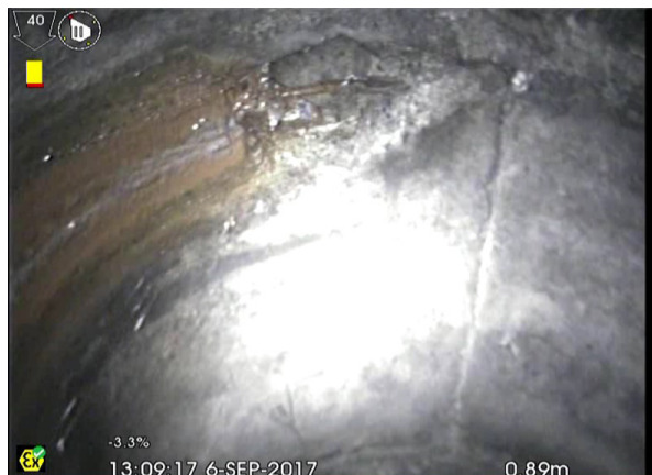
C1X_fad6a9a5-0175-48cf-aa51-6d8a3521a665_20170912_084205_694.jpg, 00:00:22, 0.89m Infiltration, dripping at 10 o'clock
