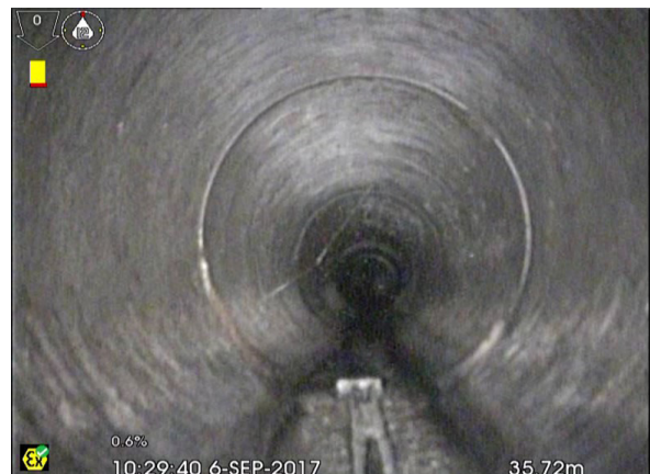
C2X_cf1d6884-148c-4efe-a6a2-4aed3da1a56c_20170912_081617_357.jpg, 00:03:25, 35.72m Other obstacles, other object in invert at 6 o'clock, 5% cross-sectional area loss
