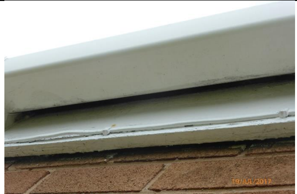
Photograph 10: Bat roost feature identified within building 6
