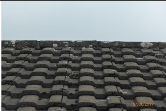
Photograph 11: Bat roost feature identified within building 7.
