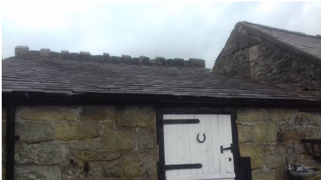
Front elevation of Outbuilding 1 (O1) showing potential in lifted/loose/missing tiles and lifted ridge tiles
