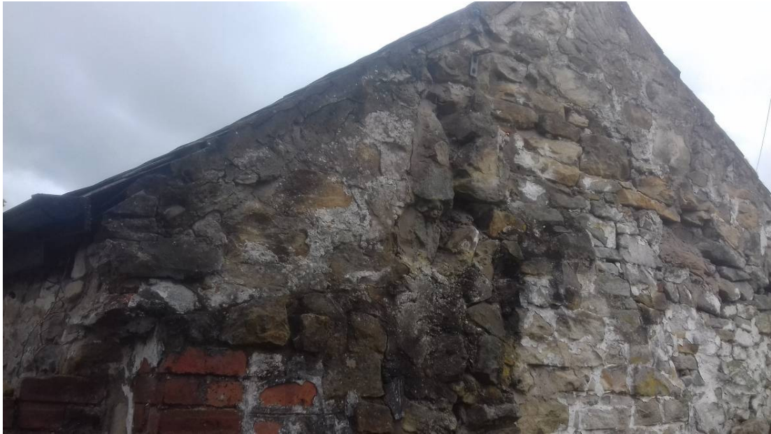
Gaps in stone work of O1
