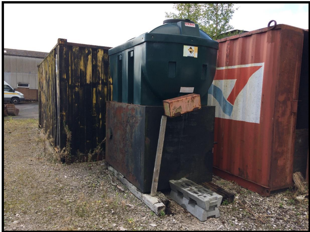
4. Fuel tank in north of the site.
