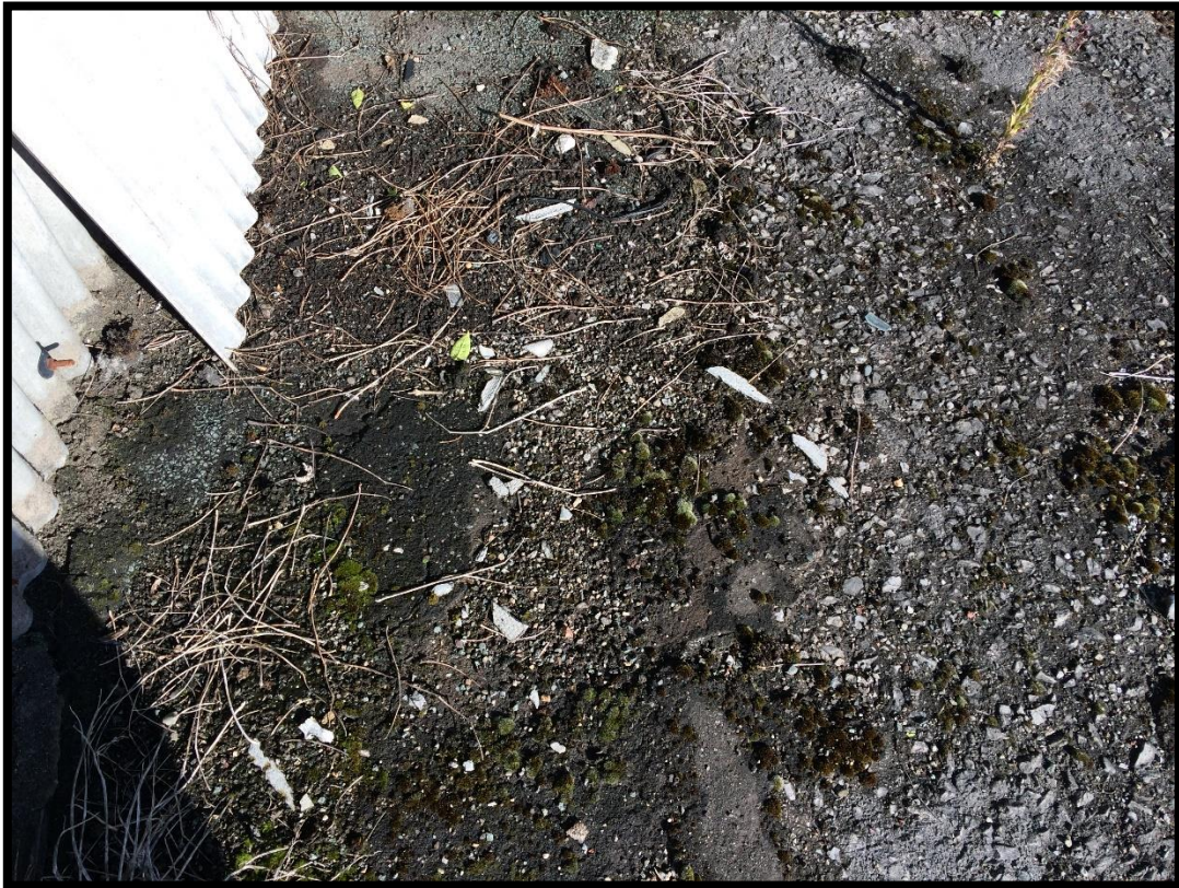
7. Potential ACMs from cladding on the buildings in the centre of the site.
