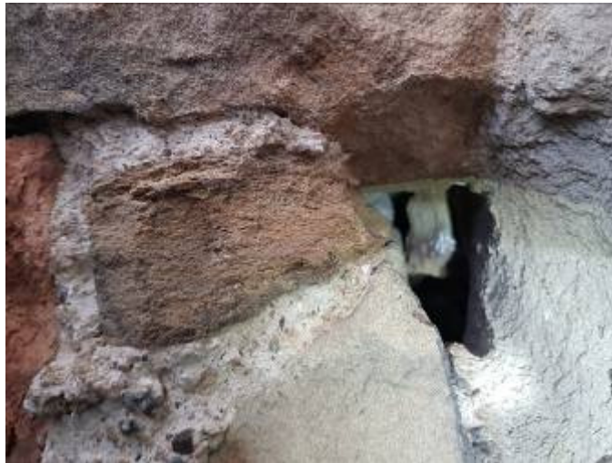
Gaps in stonework on B2
