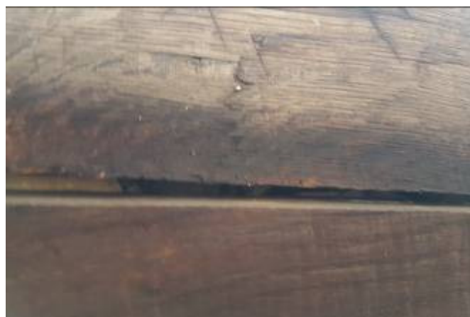
Gaps in stone lintels noted to B2
