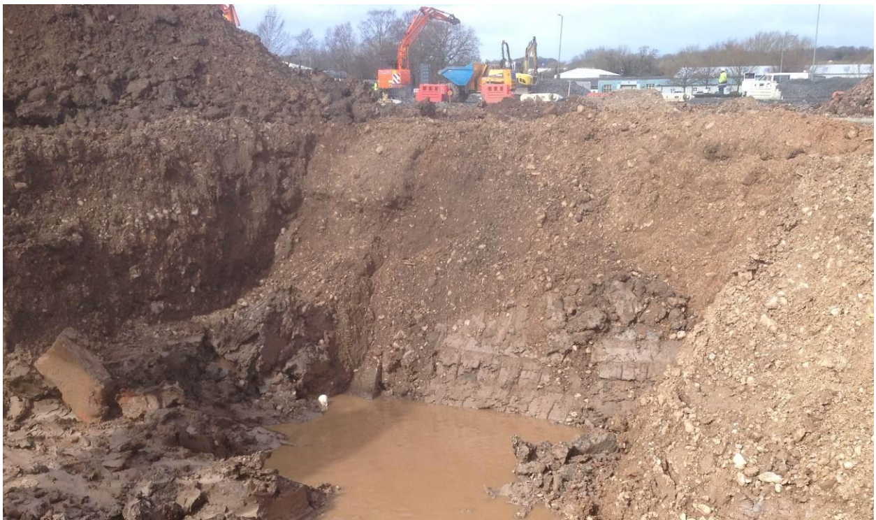
Figure 6: Water perched on top of concrete slab.
