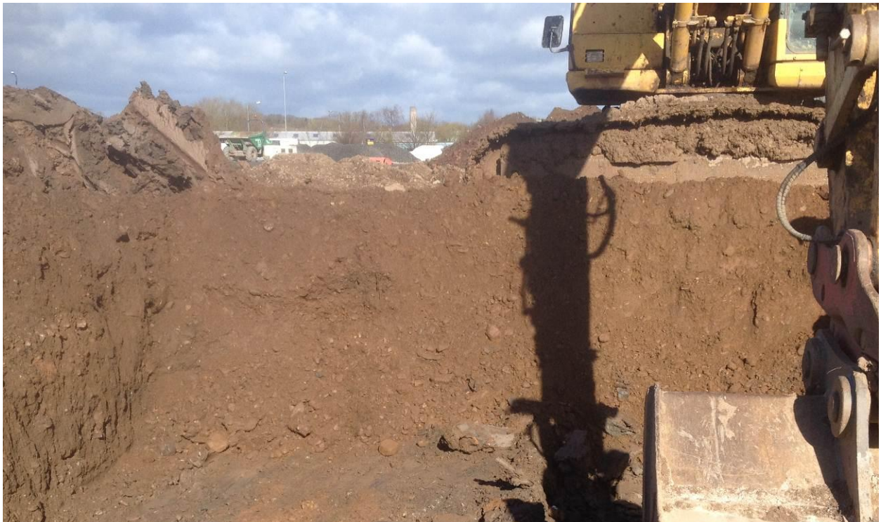
Figure 1: Northwestern edge of 'soft spot' excavation where S3 was taken.
