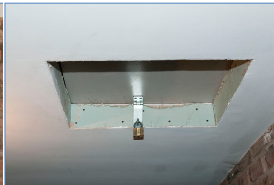
Photograph 6: Access is controlled by a separate padlock.
