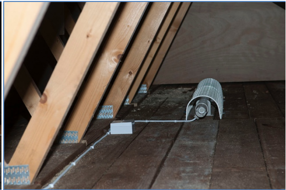
Photograph 10: The heater also appears to be functioning correctly.
