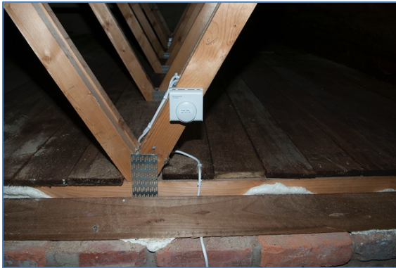
Photograph 9: The heater has a separate thermostatic control.
