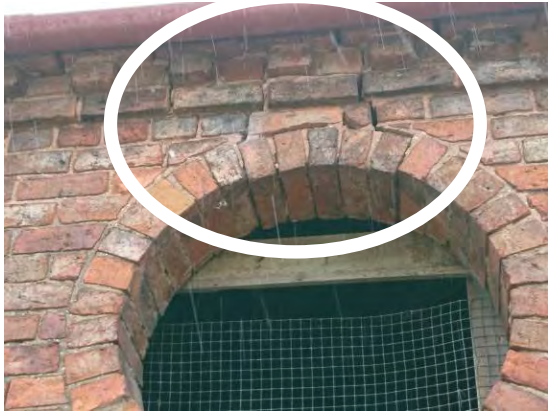
Photo 6 – Loose brickwork above opening and to arch ring.
