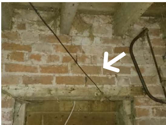
Photo 8 – Cracking above internal opening.
