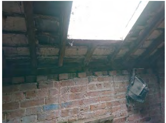
Photo 19 – Staining to sheeting.
