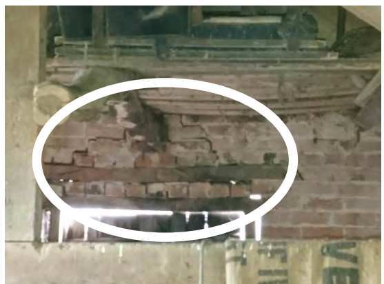
Photo 11 – Inadequate lintel and loose brickwork above opening.
