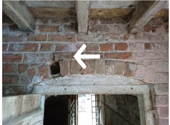
Photos 9 – Cracking above internal opening. Note missing brick.
