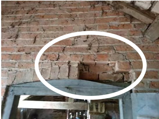
Photo 12 – Missing brickwork above opening. Note cracking above.
