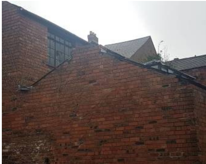
Gaps to the verge at the rear elevation
