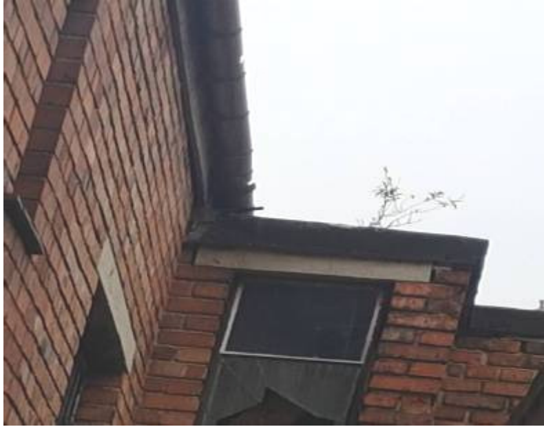
Gaps at lintel
