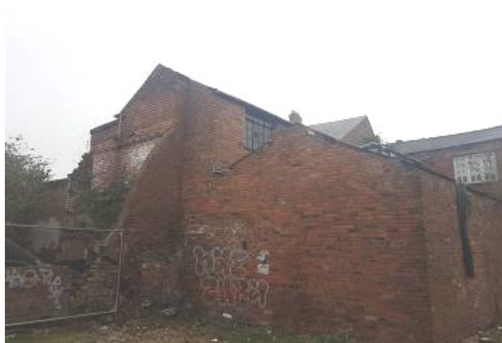
Rear elevation where partial collapse has occurred
