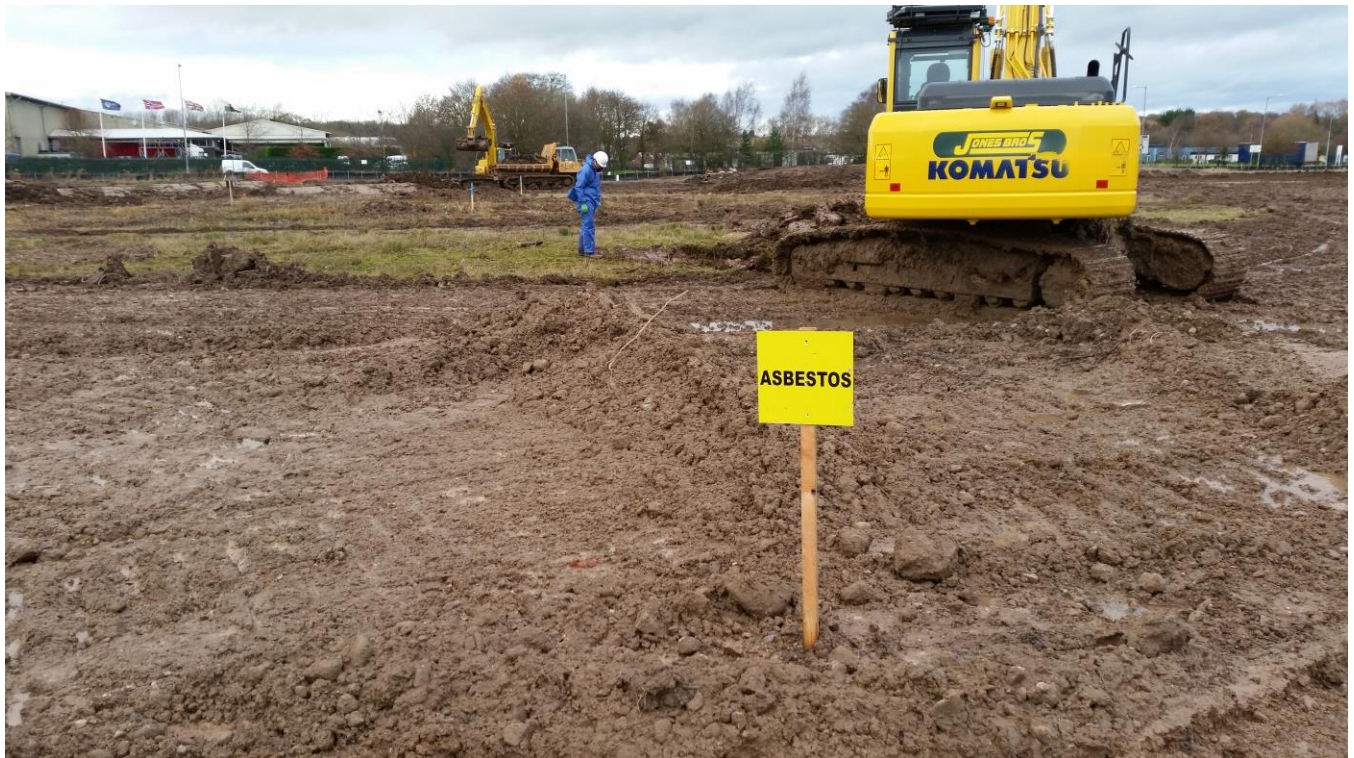
Figure 1: 2141209_133216: Area quarantined and undergoing inspection
