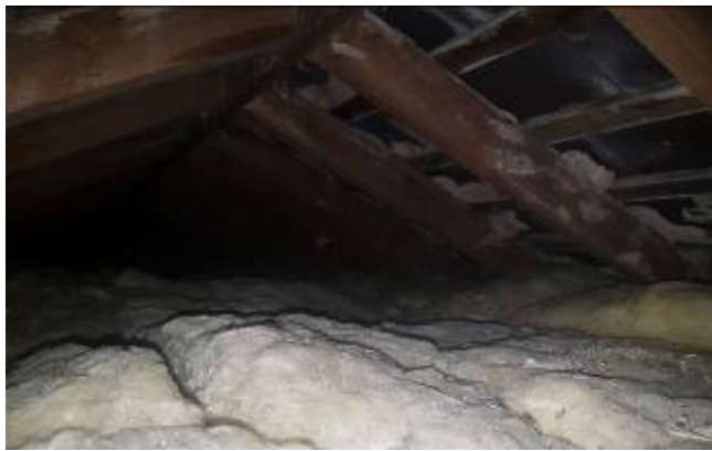
Absence of any lining visible
