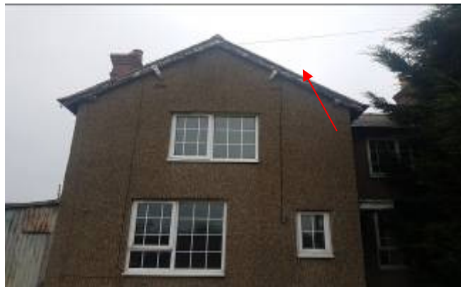
Front elevation of Newgate Farm with gap at verge visible
