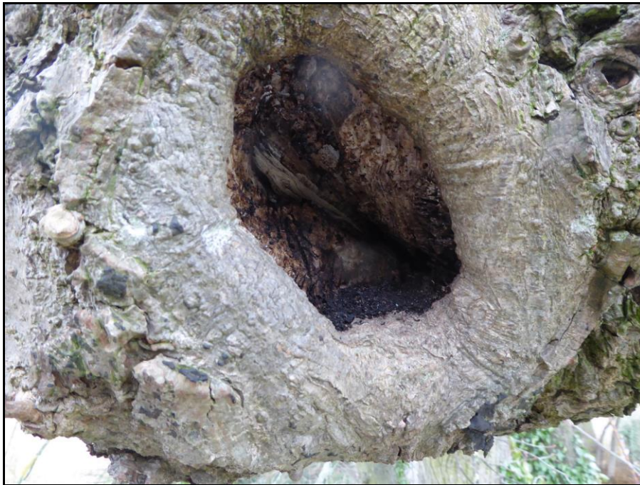
Photograph 3 showing another cavity with damp detritus
