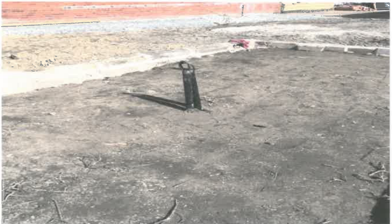
AWAITING TO BE CAPED
