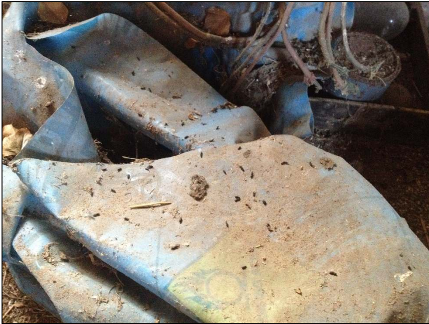
A1.7 Plate 7 – Bat droppings at TN2 within Building B1a
