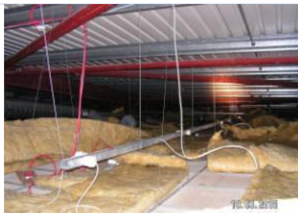
d) Above suspended ceiling, light spill from factory lights illuminates the void. No droppings observed on floor lagging.
