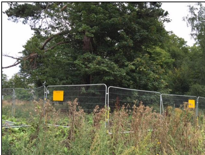
Photo 9 - Tree protective fencing around Pine tree to east - note large diameter dead wood in crown that needs to be removed
