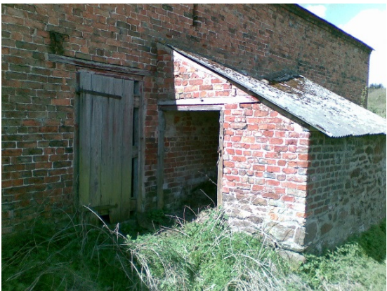
Photograph 14: Failed lean-to. To be removed
