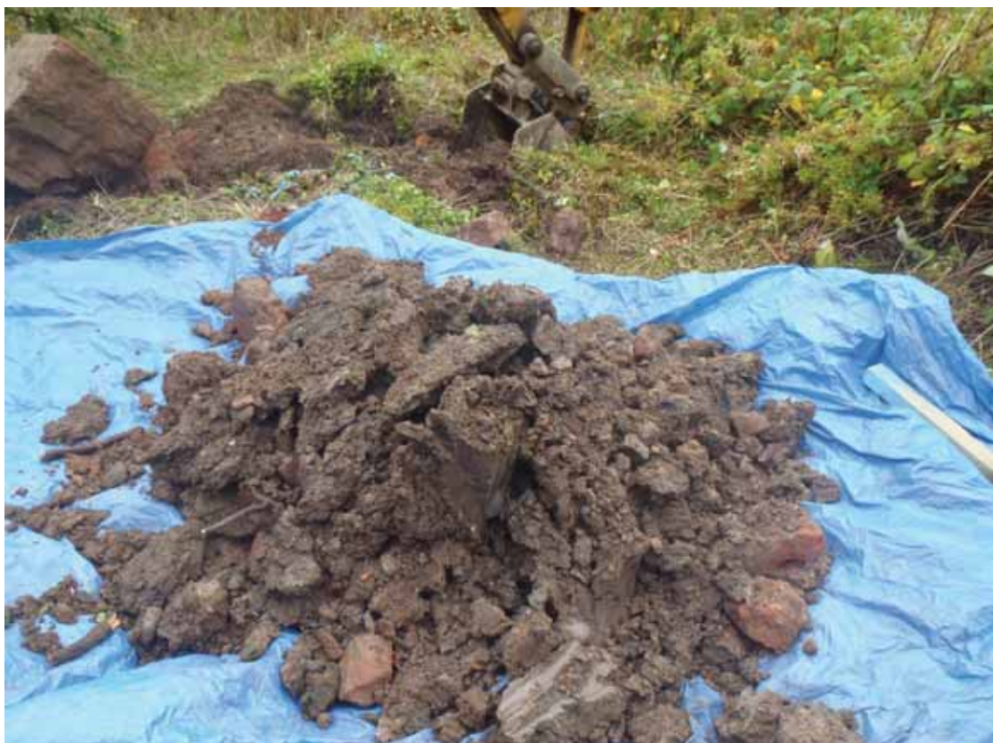
TP3: Showing fragments of brick and rocks in Made Ground
