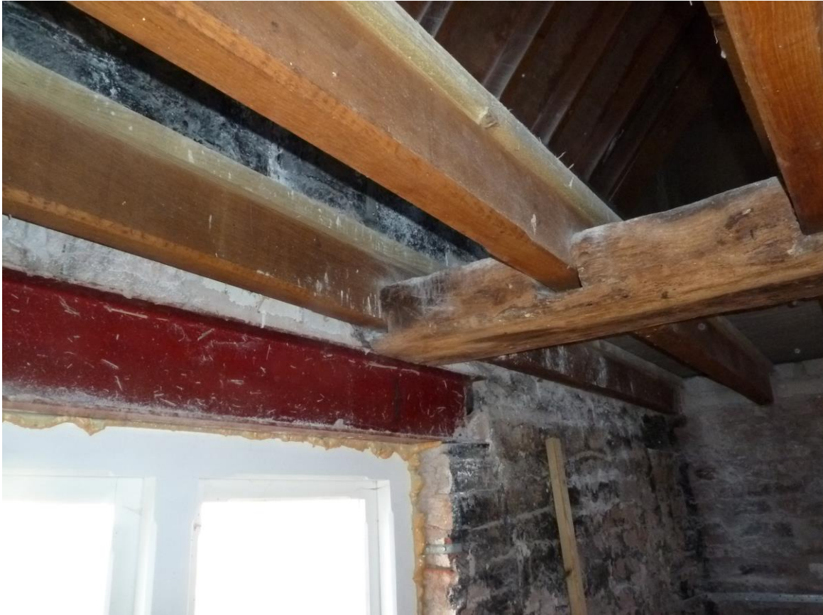
The defective main beam seated over a non-approved steel window lintol
