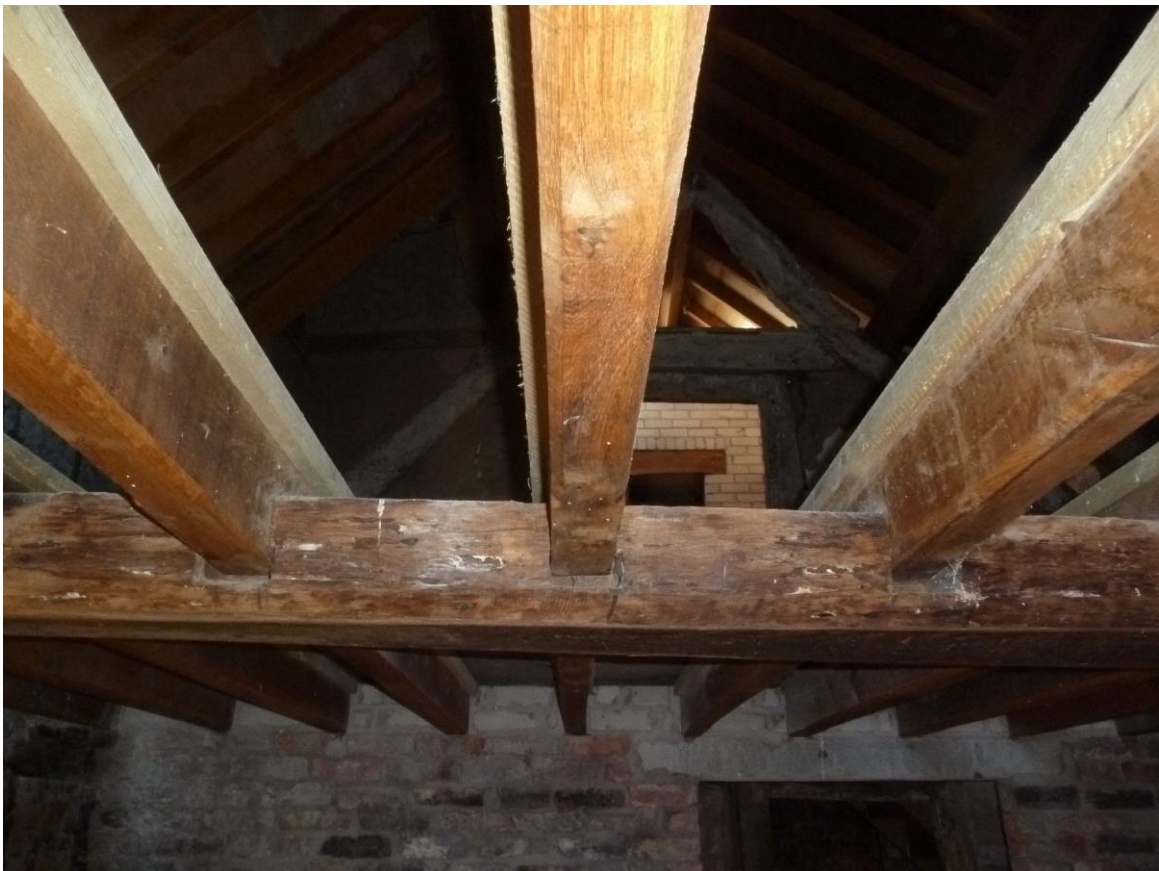
The defective main beam with previously approved new floor joists which are not bearing fully on it.
