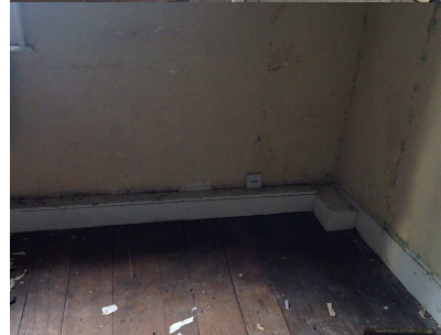
Skirting is in poor condition, missing and parts have been replaced with softwood torus, parts have been ripped out and replaced with pipe boxing
