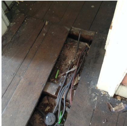
The second floor wiring is in need of stripping out and reforming
