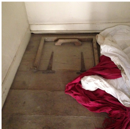
The existing second floor fire escape route is not fit for purpose. A new staircase is proposed in order to make the rooms habitable.
