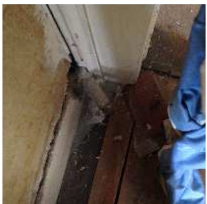
Previous services have been fitted in a poor and unsightly manner
