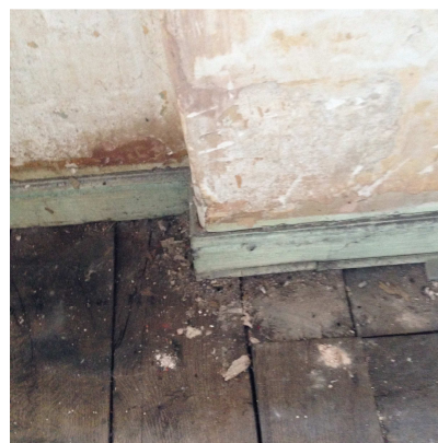
The plaster on external walls is poor
