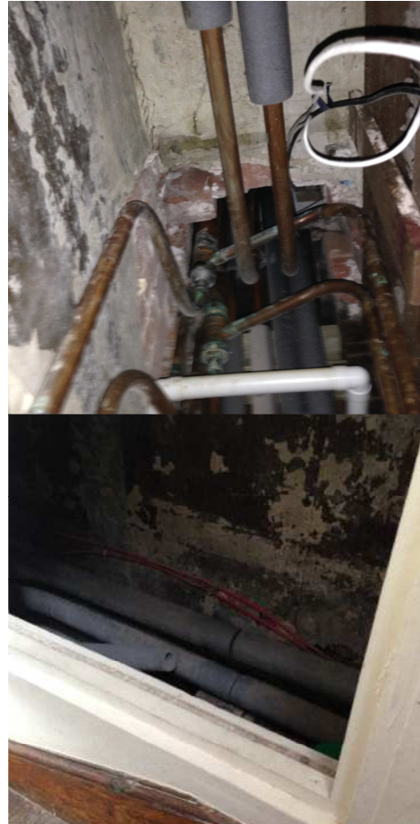
The concealed void behind the existing back staircase needs to be upgraded to 1 hour fire rating (this can be carried without affecting the finishes)
