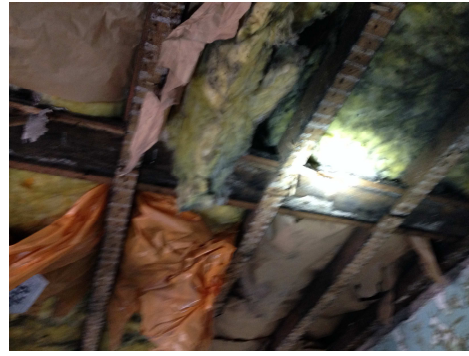
Some of the ceilings are no longer in situ
