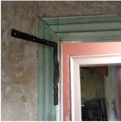
Joinery is mismatched, missing and in need of overhauling
